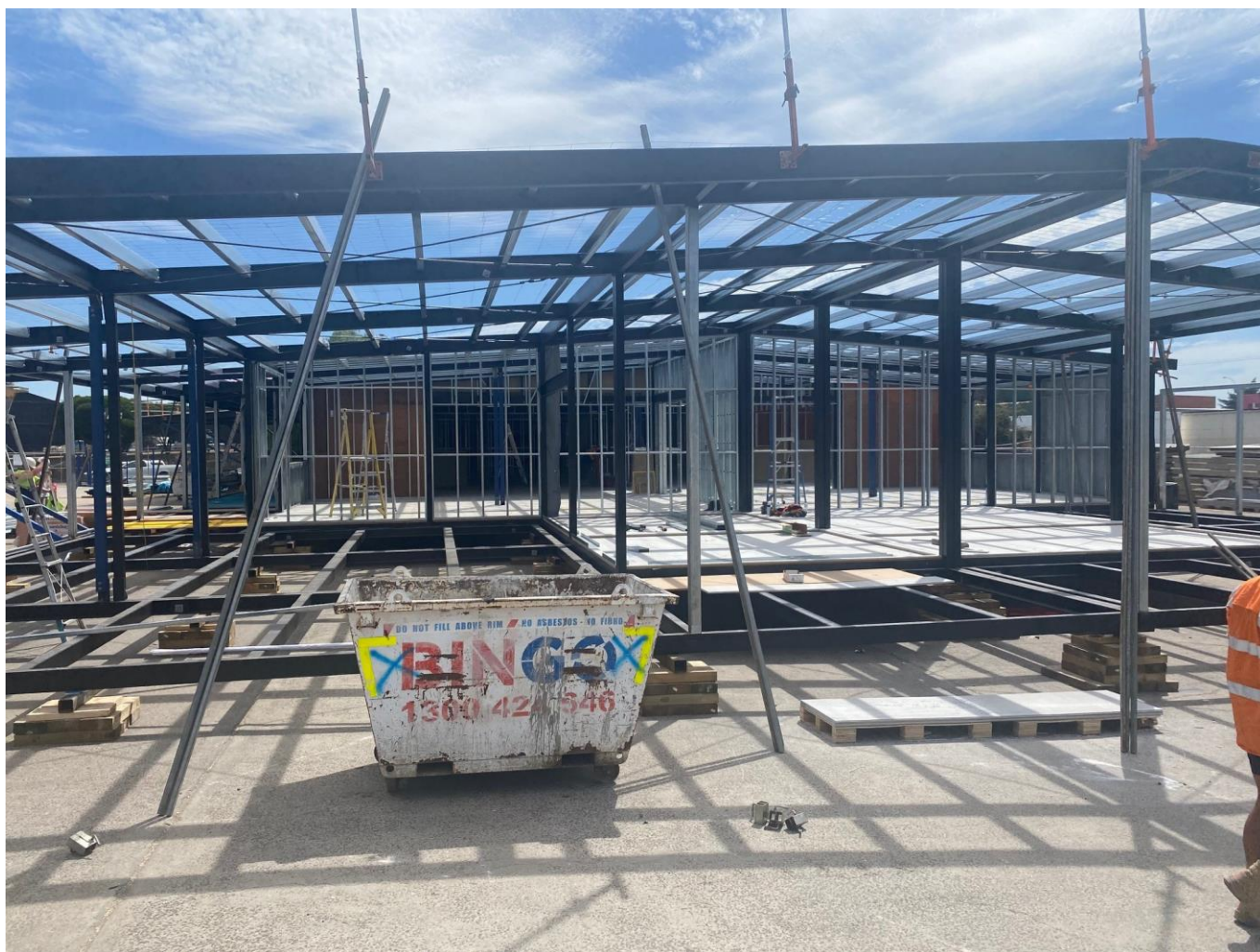
Caption: The school's structural frame is now complete. Next stage will be adding the roof and facade.
