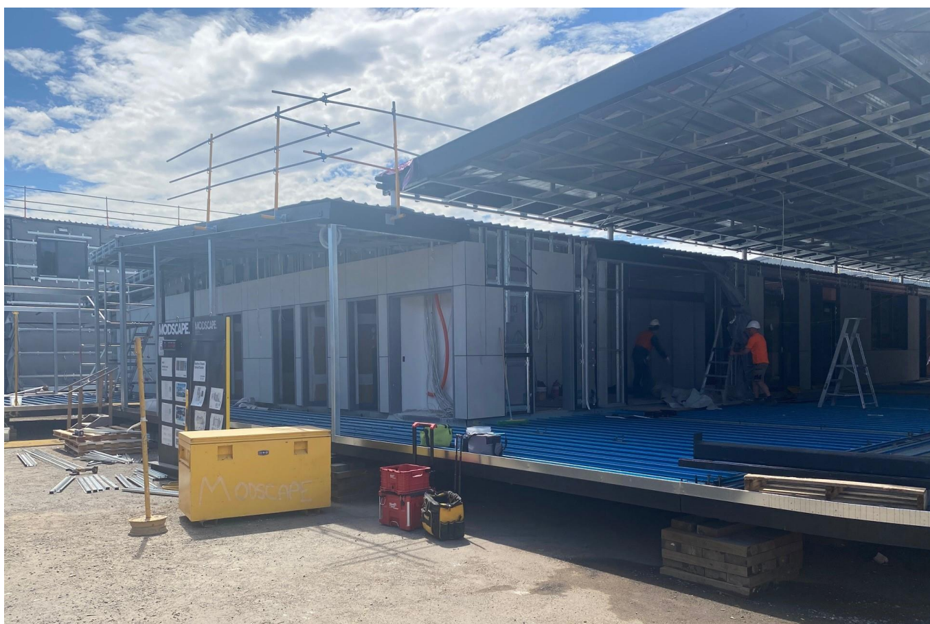
Caption: Empire Vale PS under construction. The internal services have been installed and the partition walls have been closed. Painting and final fixtures will commence shortly.
