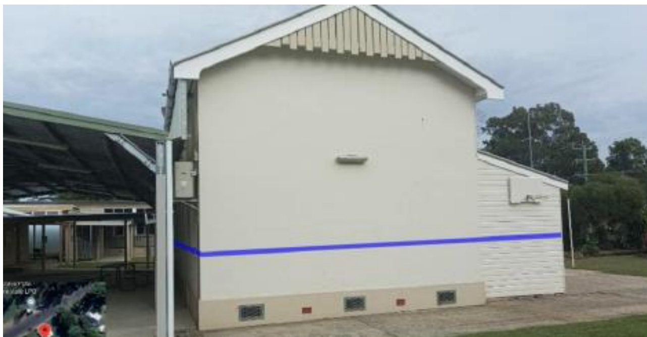
Figure 19 Building B Original school building (library) with blue line indicating the approximate height of the 2022 floods with a blue line (Source: Acor Consultants)
