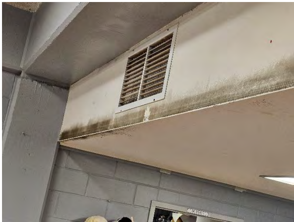
Image 9: Mould by air-conditioning duct
