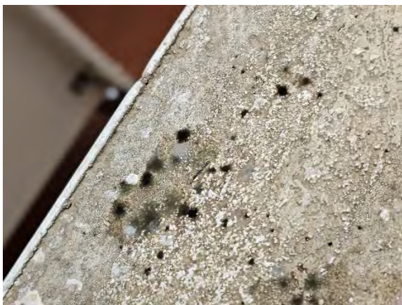
Image 5: Mould on concrete
