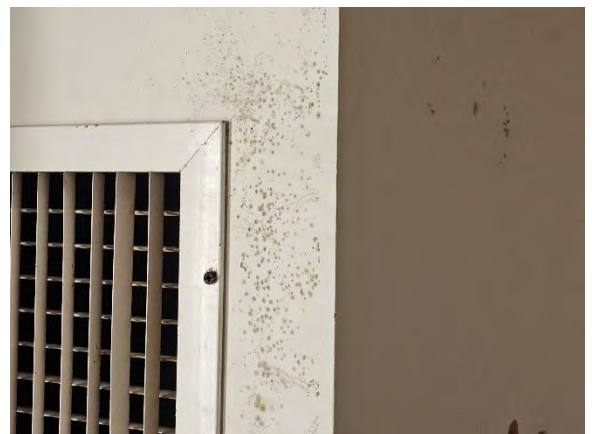
Image 6: Mould nearby air-conditioning duct
