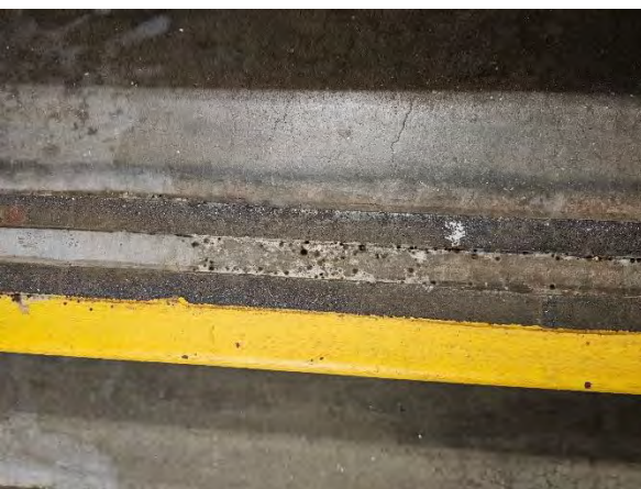
Image 41: Mould, concrete steps
