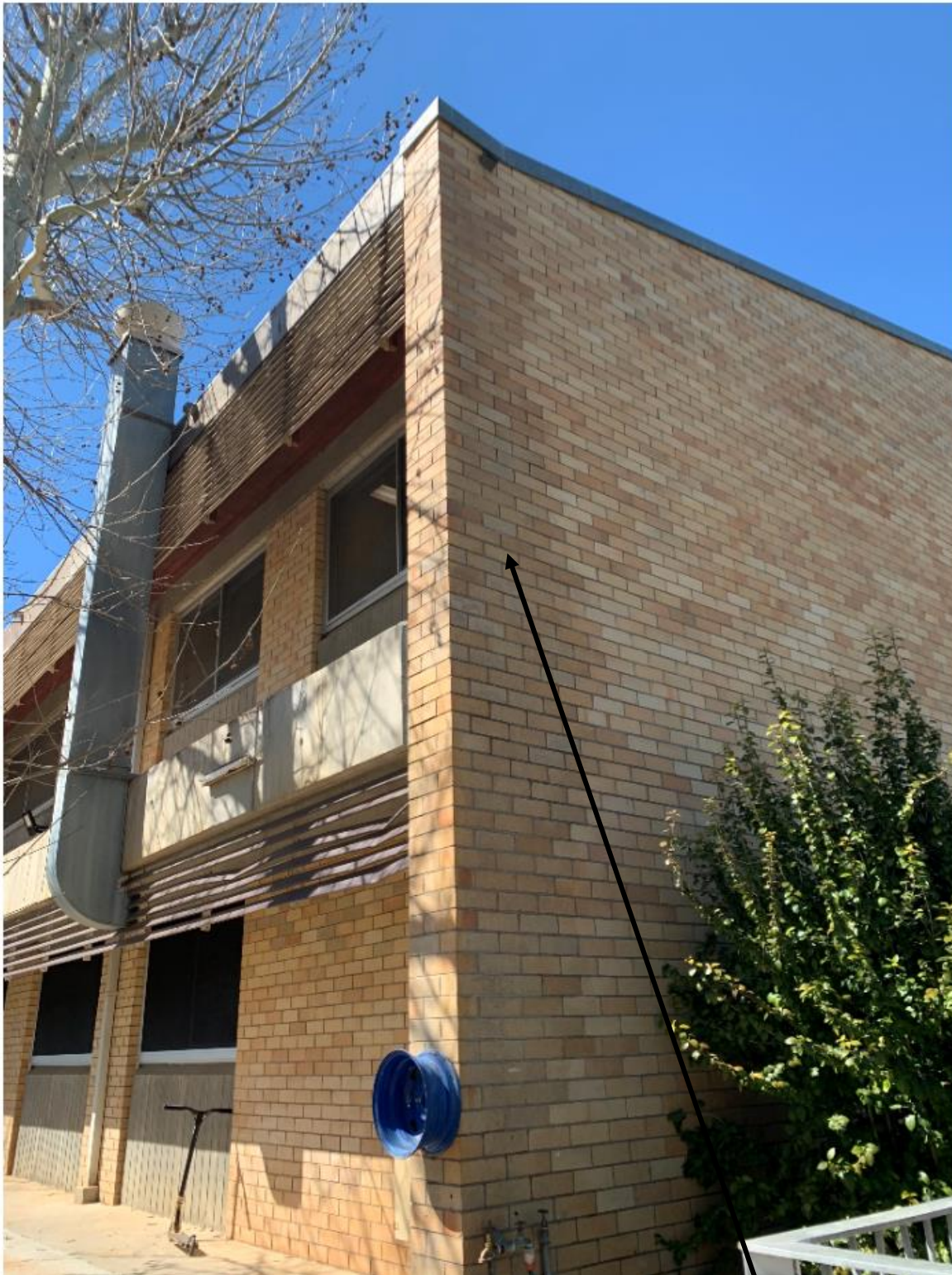
Visible damp (dark area)
