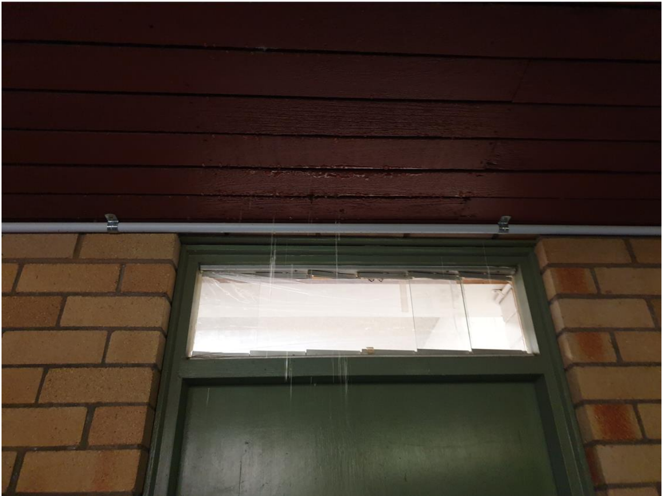
Figure 4.7: Roof leak A block in February 2020
