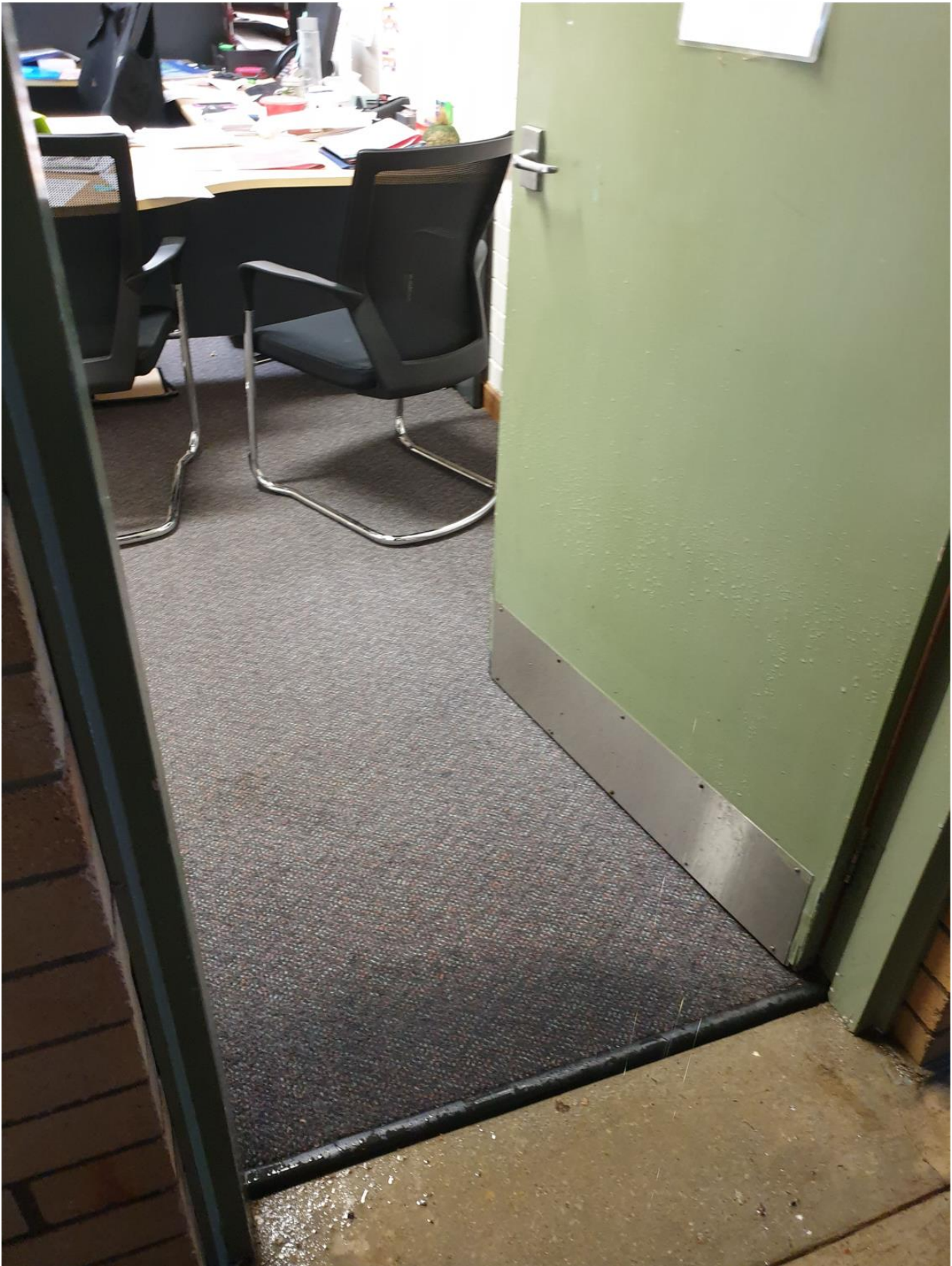
Figure 4.6: Roof leak A block in February 2020 – water damage
