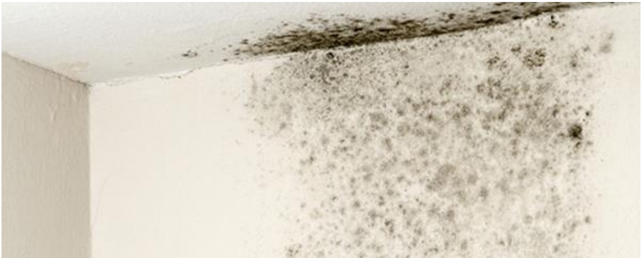
Figure 9.3: Mould growing on a damp wall
