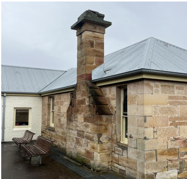
Chimneys to be restored
