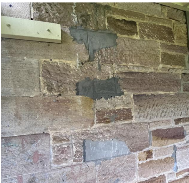
Stone to be replaced
