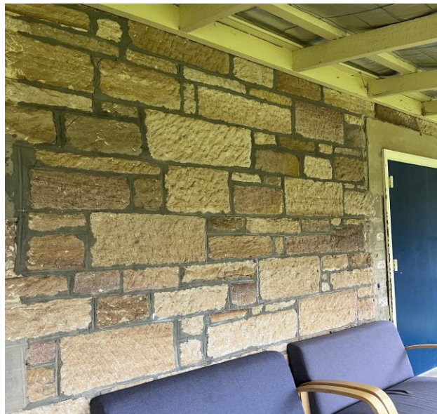
Stonework to be repointed
