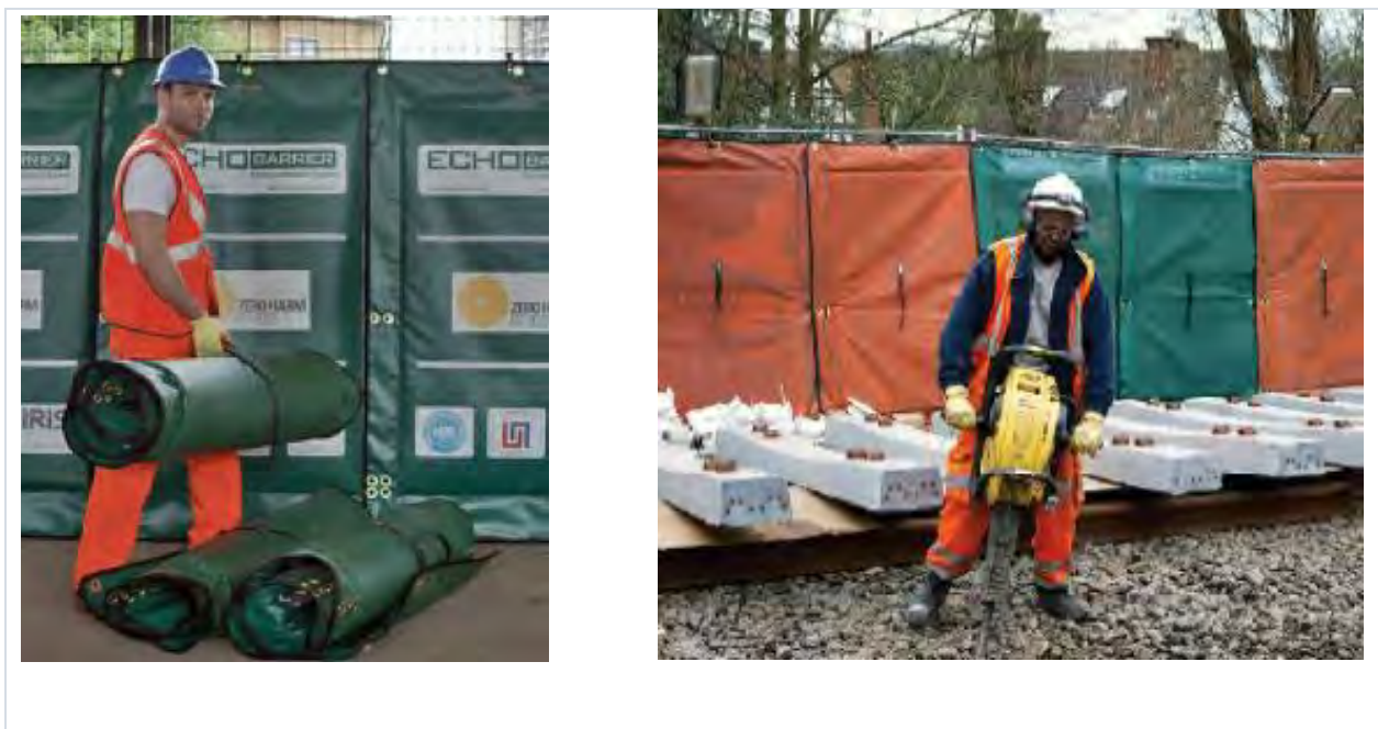
Figure 8: Photos demountable noise barriers
