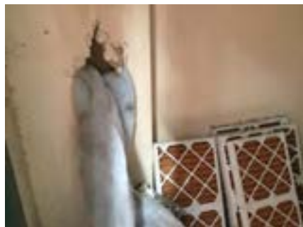
PHOTO NO.: J154351-001-PHOTO066 RESULT: SMF - POSITIVE BUILDING/LEVEL: B00E - GROUND LEVEL ROOM/LOCATION: ER0002 - PLANT ROOM - THROUGHOUT FEATURE/MATERIAL: INSULATION - INSULATION MATERIAL SAMPLE NO.: -
