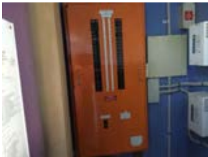
PHOTO NO.: J154351-001-PHOTO144 RESULT: ASBESTOS - PRESUMED POSITIVE BUILDING/LEVEL: B00D - LEVEL ONE ROOM/LOCATION: DR1014 - ELECTRICAL CUPBOARD - WEST FEATURE/MATERIAL: ELECTRICAL - SWITCH BOARD - COMPRESSED BITUMINOUS ELECTRICAL PANEL SAMPLE NO.: NOT SAMPLED LIVE ELECTRICAL HAZARD
