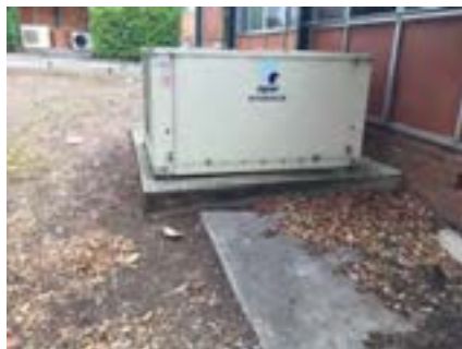
PHOTO NO.: J154351-001-PHOTO190 RESULT: ODS - POSITIVE BUILDING/LEVEL: B00A - GROUND LEVEL ROOM/LOCATION: EXTERIOR - SOUTHEAST FEATURE/MATERIAL: A/C UNIT - R22 - CHLORODIFLUOROMETHANE SAMPLE NO.: -
