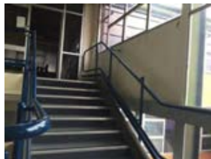
PHOTO NO.: J154351-001-PHOTO095 RESULT: ASBESTOS - POSITIVE BUILDING/LEVEL: B00E - GROUND LEVEL ROOM/LOCATION: ER1014 - STAIRWELL - WEST FEATURE/MATERIAL: INFILL PANELS - COMPRESSED CEMENT SHEETING SAMPLE NO.: PREVIOUSLY SAMPLED GREENCAP J146932-02-002-024
