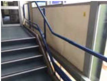
PHOTO NO.: J154351-001-PHOTO114 RESULT: ASBESTOS - POSITIVE BUILDING/LEVEL: B00B - LEVEL ONE ROOM/LOCATION: BR1019 - COVERD WALKWAY (CONNECTING BUILDING E & B) - SOUTH FEATURE/MATERIAL: INFILL PANELS - COMPRESSED CEMENT SHEETING SAMPLE NO.: PREVIOUSLY SAMPLED GREENCAP J146932-02-002-024
