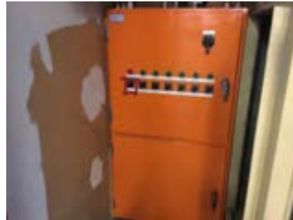
PHOTO NO.: J154351-001-PHOTO030 RESULT: ASBESTOS - PRESUMED POSITIVE BUILDING/LEVEL: B00A - GROUND LEVEL ROOM/LOCATION: AR0009 - PLANT ROOM - WEST FEATURE/MATERIAL: ELECTRICAL - SWITCH BOARD - COMPRESSED BITUMINOUS ELECTRICAL PANEL SAMPLE NO.: NOT SAMPLED LIVE ELECTRICAL HAZARD
