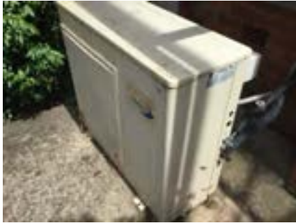
PHOTO NO.: J154351-001-PHOTO126 RESULT: ODS - POSITIVE BUILDING/LEVEL: B00B - GROUND LEVEL ROOM/LOCATION: EXTERIOR - VARIOUS THROUGHOUT FEATURE/MATERIAL: A/C UNIT - R22 - CHLORODIFLUOROMETHANE SAMPLE NO.: -
