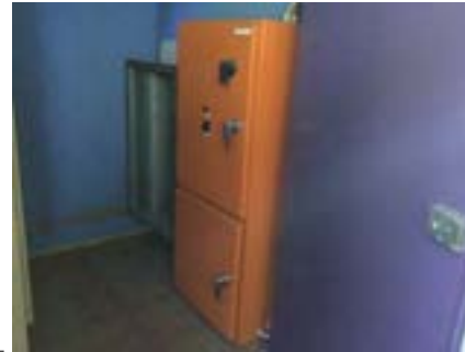
PHOTO NO.: J154351-001-PHOTO139 RESULT: ASBESTOS - PRESUMED POSITIVE BUILDING/LEVEL: B00D - LEVEL ONE ROOM/LOCATION: DR1009 - PLANT ROOM - NORTH FEATURE/MATERIAL: ELECTRICAL - SWITCH BOARD - COMPRESSED BITUMINOUS ELECTRICAL PANEL SAMPLE NO.: NOT SAMPLED HEIGHT RESTRICTED
