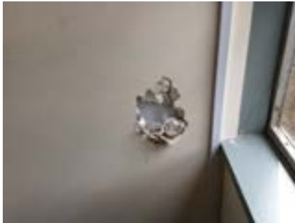
PHOTO NO.: J154351-001-PHOTO080 RESULT: SMF - POSITIVE BUILDING/LEVEL: B00E - LEVEL ONE ROOM/LOCATION: ALL ROOMS - VARIOUS THROUGHOUT FEATURE/MATERIAL: INSULATION - INSULATION MATERIAL SAMPLE NO.: -
