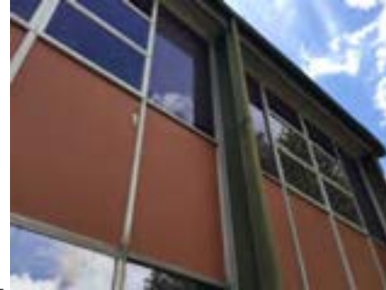
PHOTO NO.: J154351-001-PHOTO186 RESULT: ASBESTOS - POSITIVE BUILDING/LEVEL: B00D - ALL LEVELS ROOM/LOCATION: ALL AREAS - VARIOUS THROUGHOUT FEATURE/MATERIAL: INFILL PANELS - COMPRESSED CEMENT SHEETING SAMPLE NO.: PREVIOUSLY SAMPLED GREENCAP J146932-02-002-024
