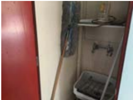
PHOTO NO.: J154351-001-PHOTO010 RESULT: SMF - POSITIVE BUILDING/LEVEL: B00K - GROUND LEVEL ROOM/LOCATION: KR0004 - CLEANERS STORE - VARIOUS THROUGHOUT FEATURE/MATERIAL: INSULATION - INSULATION MATERIAL SAMPLE NO.: -
