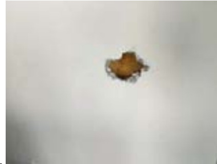
PHOTO NO.: J154351-001-PHOTO081 RESULT: SMF - POSITIVE BUILDING/LEVEL: B00E - LEVEL ONE ROOM/LOCATION: ALL ROOMS - VARIOUS THROUGHOUT FEATURE/MATERIAL: INSULATION - INSULATION MATERIAL SAMPLE NO.: -
