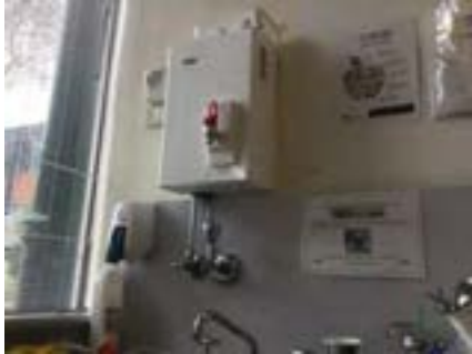
PHOTO NO.: J154351-001-PHOTO026 RESULT: SMF - PRESUMED POSITIVE BUILDING/LEVEL: B00A - GROUND LEVEL ROOM/LOCATION: AR0005 - KITCHEN - ABOVE SINK FEATURE/MATERIAL: HOT WATER SERVICE INSULATION - INSULATION MATERIAL SAMPLE NO.: -
