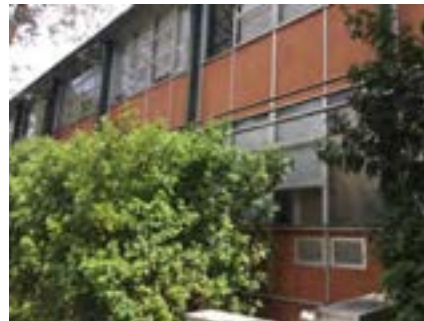
PHOTO NO.: J154351-001-PHOTO129 RESULT: ASBESTOS - POSITIVE BUILDING/LEVEL: B00B - ALL LEVELS ROOM/LOCATION: ALL AREAS - VARIOUS THROUGHOUT FEATURE/MATERIAL: INFILL PANELS - COMPRESSED CEMENT SHEETING SAMPLE NO.: PREVIOUSLY SAMPLED GREENCAP J146932-02-002-024
