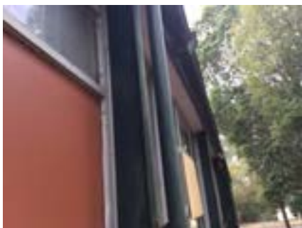
PHOTO NO.: J154351-001-PHOTO036 RESULT: ASBESTOS - POSITIVE BUILDING/LEVEL: B00A - GROUND LEVEL ROOM/LOCATION: EXTERIOR - VARIOUS THROUGHOUT FEATURE/MATERIAL: EAVES - FIBRE CEMENT SHEETING SAMPLE NO.: J154351-001-010
