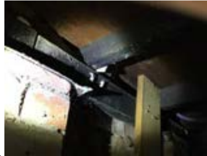
PHOTO NO.: J154351-001-PHOTO046 RESULT: ASBESTOS - POSITIVE BUILDING/LEVEL: B00A - SUB-FLOOR ROOM/LOCATION: ALL AREAS - VARIOUS THROUGHOUT FEATURE/MATERIAL: PACKER - FIBRE CEMENT SHEETING SAMPLE NO.: J154351-001-014
