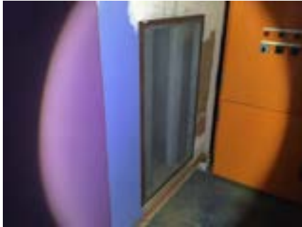
PHOTO NO.: J154351-001-PHOTO149 RESULT: SMF - POSITIVE BUILDING/LEVEL: B00D - LEVEL ONE ROOM/LOCATION: DR1019 - PLANT ROOM - NORTH FEATURE/MATERIAL: DUCTWORK INSULATION - INSULATION MATERIAL SAMPLE NO.: -
