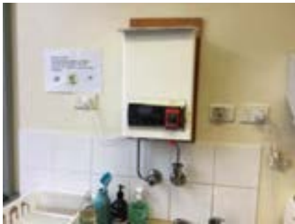
PHOTO NO.: J154351-001-PHOTO174 RESULT: SMF - PRESUMED POSITIVE BUILDING/LEVEL: B00D - GROUND LEVEL ROOM/LOCATION: DR0019 - STAFF KITCHEN/LUNCH ROOM - ABOVE SINK FEATURE/MATERIAL: HOT WATER SERVICE INSULATION - INSULATION MATERIAL SAMPLE NO.: -
