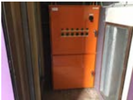
PHOTO NO.: J154351-001-PHOTO103 RESULT: ASBESTOS - PRESUMED POSITIVE BUILDING/LEVEL: B00E - LEVEL ONE ROOM/LOCATION: ER1004 - PLANT ROOM - EAST FEATURE/MATERIAL: ELECTRICAL - SWITCH BOARD - COMPRESSED BITUMINOUS ELECTRICAL PANEL SAMPLE NO.: NOT SAMPLED LIVE ELECTRICAL HAZARD
