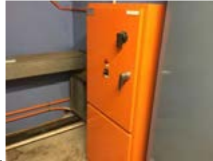
PHOTO NO.: J154351-001-PHOTO179 RESULT: ASBESTOS - PRESUMED POSITIVE BUILDING/LEVEL: B00D - GROUND LEVEL ROOM/LOCATION: DR0023 - PLANT ROOM - NORTH FEATURE/MATERIAL: ELECTRICAL - SWITCH BOARD - COMPRESSED BITUMINOUS ELECTRICAL PANEL SAMPLE NO.: NOT SAMPLED HEIGHT RESTRICTED
