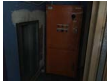
PHOTO NO.: J154351-001-PHOTO148 RESULT: ASBESTOS - PRESUMED POSITIVE BUILDING/LEVEL: B00D - LEVEL ONE ROOM/LOCATION: DR1019 - PLANT ROOM - EAST FEATURE/MATERIAL: ELECTRICAL - SWITCH BOARD - COMPRESSED BITUMINOUS ELECTRICAL PANEL SAMPLE NO.: NOT SAMPLED HEIGHT RESTRICTED
