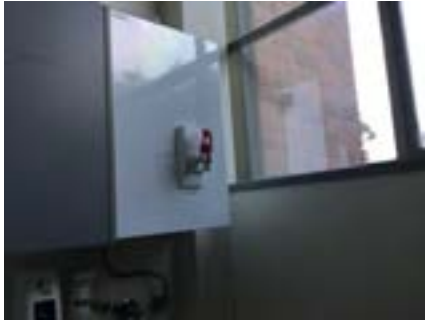
PHOTO NO.: J154351-001-PHOTO156 RESULT: SMF - PRESUMED POSITIVE BUILDING/LEVEL: B00D - LEVEL ONE ROOM/LOCATION: DR1002 - KITCHEN - ABOVE SINK FEATURE/MATERIAL: HOT WATER SERVICE INSULATION - INSULATION MATERIAL SAMPLE NO.: -
