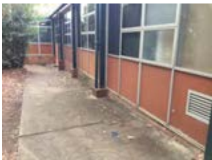
PHOTO NO.: J154351-001-PHOTO015 RESULT: ASBESTOS - POSITIVE BUILDING/LEVEL: B00A - GROUND LEVEL ROOM/LOCATION: EXTERIOR - VARIOUS THROUGHOUT FEATURE/MATERIAL: INFILL PANELS - COMPRESSED CEMENT SHEETING SAMPLE NO.: PREVIOUSLY SAMPLED GREENCAP J146932-02-002-024
