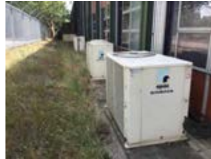
PHOTO NO.: J154351-001-PHOTO192 RESULT: ODS - POSITIVE BUILDING/LEVEL: B00D - GROUND LEVEL ROOM/LOCATION: EXTERIOR - VARIOUS THROUGHOUT FEATURE/MATERIAL: A/C UNIT - R22 - CHLORODIFLUOROMETHANE SAMPLE NO.: -
