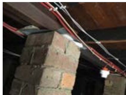
PHOTO NO.: J154351-001-PHOTO102 RESULT: ASBESTOS - POSITIVE BUILDING/LEVEL: B00E - SUB-FLOOR ROOM/LOCATION: ALL AREAS - VARIOUS THROUGHOUT FEATURE/MATERIAL: PACKER - FIBRE CEMENT SHEETING SAMPLE NO.: J154351-001-032
