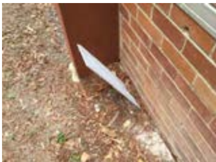
PHOTO NO.: J154351-001-PHOTO038 RESULT: ASBESTOS - PRESUMED POSITIVE BUILDING/LEVEL: B00A - GROUND LEVEL ROOM/LOCATION: EXTERIOR - NORTHEAST FEATURE/MATERIAL: EAVES - FIBRE CEMENT SHEETING SAMPLE NO.: SIMILAR TO: J154351-001-010
