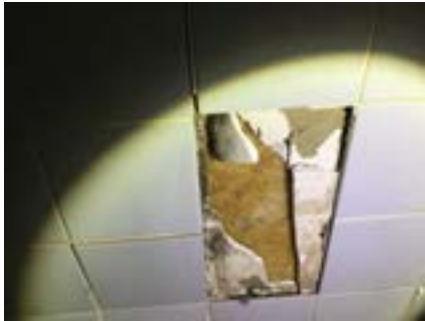
PHOTO NO.: J154351-001-PHOTO004 RESULT: SMF - POSITIVE BUILDING/LEVEL: B00K - GROUND LEVEL ROOM/LOCATION: KR0008 - MENS SHOWER - VARIOUS THROUGHOUT FEATURE/MATERIAL: INSULATION - INSULATION MATERIAL SAMPLE NO.: -
