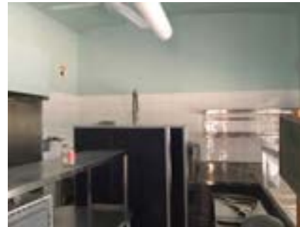
PHOTO NO.: J154351-001-PHOTO011 RESULT: SMF - POSITIVE BUILDING/LEVEL: B00K - GROUND LEVEL ROOM/LOCATION: KR0005 - KITCHEN - VARIOUS THROUGHOUT FEATURE/MATERIAL: INSULATION - INSULATION MATERIAL SAMPLE NO.: -
