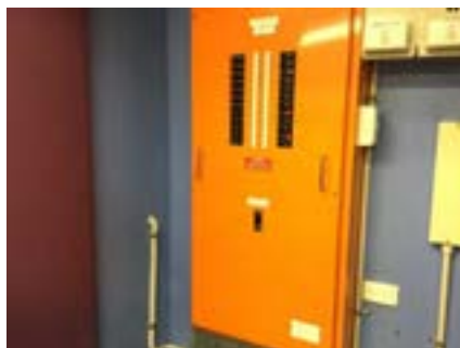
PHOTO NO.: J154351-001-PHOTO019 RESULT: ASBESTOS - PRESUMED POSITIVE BUILDING/LEVEL: B00A - GROUND LEVEL ROOM/LOCATION: AR0003 - ELECTRICAL CUPBOARD - SOUTH FEATURE/MATERIAL: ELECTRICAL - SWITCH BOARD - COMPRESSED BITUMINOUS ELECTRICAL PANEL SAMPLE NO.: NOT SAMPLED LIVE ELECTRICAL HAZARD
