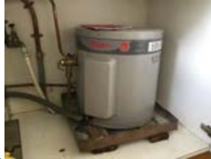
PHOTO NO.: J154351-001-PHOTO025 RESULT: SMF - PRESUMED POSITIVE BUILDING/LEVEL: B00A - GROUND LEVEL ROOM/LOCATION: AR0005 - KITCHEN - BELOW SINK FEATURE/MATERIAL: HOT WATER SERVICE INSULATION - INSULATION MATERIAL SAMPLE NO.: -
