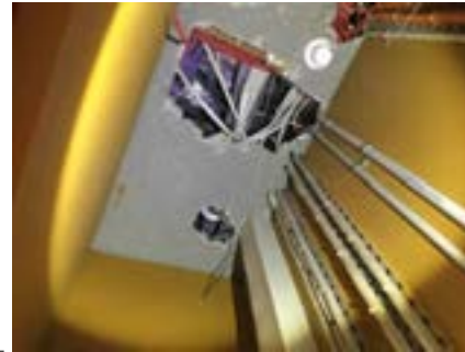
PHOTO NO.: J154351-001-PHOTO118 RESULT: SMF - POSITIVE BUILDING/LEVEL: B00B - LEVEL ONE ROOM/LOCATION: ALL ROOMS - ABOVE CEILING FEATURE/MATERIAL: INSULATION - SARKING INSULATION SAMPLE NO.: -
