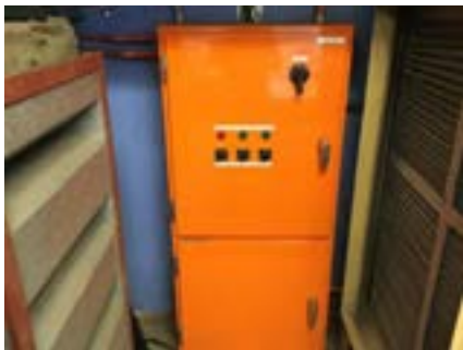
PHOTO NO.: J154351-001-PHOTO169 RESULT: ASBESTOS - PRESUMED POSITIVE BUILDING/LEVEL: B00D - GROUND LEVEL ROOM/LOCATION: DR0017 - PLANT ROOM - EAST FEATURE/MATERIAL: ELECTRICAL - SWITCH BOARD - COMPRESSED BITUMINOUS ELECTRICAL PANEL SAMPLE NO.: NOT SAMPLED LIVE ELECTRICAL HAZARD
