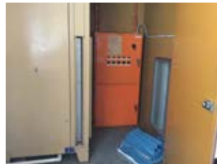
PHOTO NO.: J154351-001-PHOTO120 RESULT: ASBESTOS - PRESUMED POSITIVE BUILDING/LEVEL: B00B - LEVEL ONE ROOM/LOCATION: BR1003 - PLANT ROOM - EAST FEATURE/MATERIAL: ELECTRICAL - SWITCH BOARD - COMPRESSED BITUMINOUS ELECTRICAL PANEL SAMPLE NO.: NOT SAMPLED LIVE ELECTRICAL HAZARD
