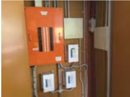
PHOTO NO.: J154351-001-PHOTO119 RESULT: ASBESTOS - PRESUMED POSITIVE BUILDING/LEVEL: B00B - LEVEL ONE ROOM/LOCATION: BR1004 - ELECTRICAL CUPBOARD - NORTH FEATURE/MATERIAL: ELECTRICAL - SWITCH BOARD - COMPRESSED BITUMINOUS ELECTRICAL PANEL SAMPLE NO.: NOT SAMPLED LIVE ELECTRICAL HAZARD
