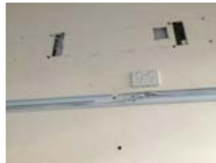
PHOTO NO.: J154351-001-PHOTO151 RESULT: SMF - POSITIVE BUILDING/LEVEL: B00D - LEVEL ONE ROOM/LOCATION: ALL ROOMS - VARIOUS THROUGHOUT FEATURE/MATERIAL: INSULATION - INSULATION MATERIAL SAMPLE NO.: -
