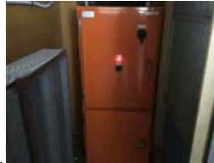
PHOTO NO.: J154351-001-PHOTO123 RESULT: ASBESTOS - PRESUMED POSITIVE BUILDING/LEVEL: B00B - LEVEL ONE ROOM/LOCATION: BR1014 - PLANT ROOM - WEST FEATURE/MATERIAL: ELECTRICAL - SWITCH BOARD - COMPRESSED BITUMINOUS ELECTRICAL PANEL SAMPLE NO.: NOT SAMPLED LIVE ELECTRICAL HAZARD
