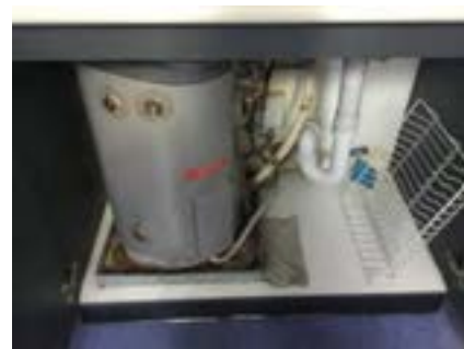
PHOTO NO.: J154351-001-PHOTO163 RESULT: SMF - PRESUMED POSITIVE BUILDING/LEVEL: B00D - GROUND LEVEL ROOM/LOCATION: DR0001 - KITCHEN - BELOW SINK FEATURE/MATERIAL: HOT WATER SERVICE INSULATION - INSULATION MATERIAL SAMPLE NO.: -
