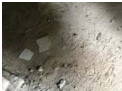
PHOTO NO.: J154351-001-PHOTO104 RESULT: ASBESTOS - PRESUMED POSITIVE BUILDING/LEVEL: B00E - SUB-FLOOR ROOM/LOCATION: ALL AREAS - VARIOUS THROUGHOUT FEATURE/MATERIAL: DEBRIS - FIBRE CEMENT SHEETING SAMPLE NO.: SIMILAR TO: J154351-001-032
