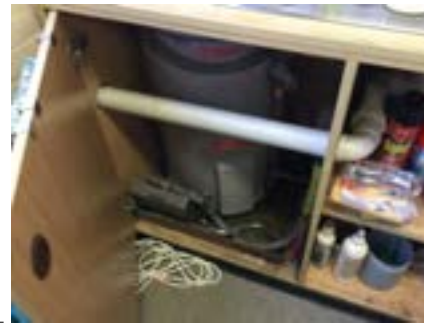
PHOTO NO.: J154351-001-PHOTO173 RESULT: SMF - PRESUMED POSITIVE BUILDING/LEVEL: B00D - GROUND LEVEL ROOM/LOCATION: DR0019 - STAFF KITCHEN/LUNCH ROOM - BELOW SINK FEATURE/MATERIAL: HOT WATER SERVICE INSULATION - INSULATION MATERIAL SAMPLE NO.: -
