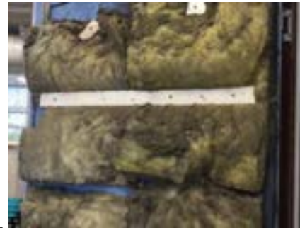
PHOTO NO.: J154351-001-PHOTO167 RESULT: SMF - POSITIVE BUILDING/LEVEL: B00D - GROUND LEVEL ROOM/LOCATION: DR0017 - PLANT ROOM - VARIOUS THROUGHOUT FEATURE/MATERIAL: INSULATION - INSULATION MATERIAL SAMPLE NO.: -
