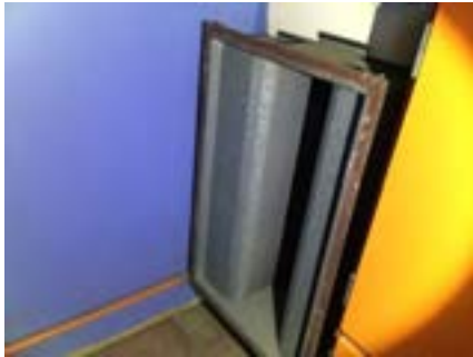
PHOTO NO.: J154351-001-PHOTO141 RESULT: SMF - POSITIVE BUILDING/LEVEL: B00D - LEVEL ONE ROOM/LOCATION: DR1009 - PLANT ROOM - NORTH FEATURE/MATERIAL: DUCTWORK INSULATION - INSULATION MATERIAL SAMPLE NO.: -
