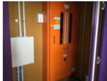
PHOTO NO.: J154351-001-PHOTO107 RESULT: ASBESTOS - PRESUMED POSITIVE BUILDING/LEVEL: B00B - LEVEL ONE ROOM/LOCATION: BR1021 - ELECTRICAL CUPBOARD(WITHIN KITCHEN) - SOUTH FEATURE/MATERIAL: ELECTRICAL - SWITCH BOARD - COMPRESSED BITUMINOUS ELECTRICAL PANEL SAMPLE NO.: NOT SAMPLED LIVE ELECTRICAL HAZARD
