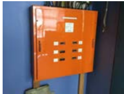
PHOTO NO.: J154351-001-PHOTO170 RESULT: ASBESTOS - PRESUMED POSITIVE BUILDING/LEVEL: B00D - GROUND LEVEL ROOM/LOCATION: DR0016 - ELECTRICAL CUPBOARD - SOUTH FEATURE/MATERIAL: ELECTRICAL - SWITCH BOARD - COMPRESSED BITUMINOUS ELECTRICAL PANEL SAMPLE NO.: NOT SAMPLED LIVE ELECTRICAL HAZARD
