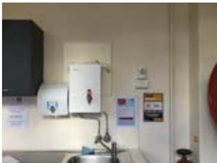
PHOTO NO.: J154351-001-PHOTO164 RESULT: SMF - PRESUMED POSITIVE BUILDING/LEVEL: B00D - GROUND LEVEL ROOM/LOCATION: DR0001 - KITCHEN - ABOVE SINK FEATURE/MATERIAL: HOT WATER SERVICE INSULATION - INSULATION MATERIAL SAMPLE NO.: -
