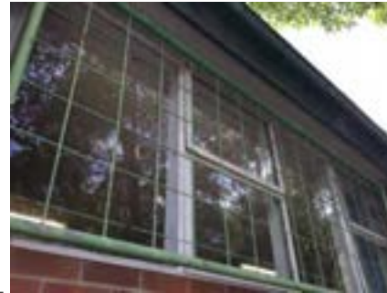
PHOTO NO.: J154351-001-PHOTO188 RESULT: ASBESTOS - PRESUMED POSITIVE BUILDING/LEVEL: B00D - LEVEL ONE ROOM/LOCATION: ALL AREAS - VARIOUS THROUGHOUT FEATURE/MATERIAL: EAVES - FIBRE CEMENT SHEETING SAMPLE NO.: NOT SAMPLED HEIGHT RESTRICTED
