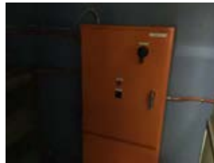
PHOTO NO.: J154351-001-PHOTO176 RESULT: ASBESTOS - PRESUMED POSITIVE BUILDING/LEVEL: B00D - GROUND LEVEL ROOM/LOCATION: DR0022 - PLANT ROOM - WEST FEATURE/MATERIAL: ELECTRICAL - SWITCH BOARD - COMPRESSED BITUMINOUS ELECTRICAL PANEL SAMPLE NO.: NOT SAMPLED HEIGHT RESTRICTED
