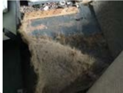
PHOTO NO.: J154351-001-PHOTO158 RESULT: ASBESTOS - POSITIVE BUILDING/LEVEL: B00D - GROUND LEVEL ROOM/LOCATION: DR0007 - SCANN/RECORDS STORAGE - THROUGHOUT FEATURE/MATERIAL: FLOOR COVERING - VINYL TILES & ADHESIVE SAMPLE NO.: J154351-001-049
