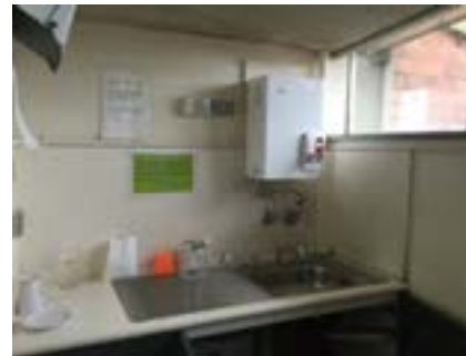
PHOTO NO.: J154351-001-PHOTO105 RESULT: SMF - PRESUMED POSITIVE BUILDING/LEVEL: B00B - LEVEL ONE ROOM/LOCATION: BR1020 - KITCHEN - ABOVE SINK FEATURE/MATERIAL: HOT WATER SERVICE INSULATION - INSULATION MATERIAL SAMPLE NO.: -
