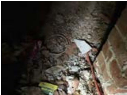
PHOTO NO.: J154351-001-PHOTO048 RESULT: ASBESTOS - POSITIVE BUILDING/LEVEL: B00A - SUB-FLOOR ROOM/LOCATION: ALL AREAS - VARIOUS THROUGHOUT FEATURE/MATERIAL: DEBRIS - FIBRE CEMENT SHEETING SAMPLE NO.: J154351-001-015
