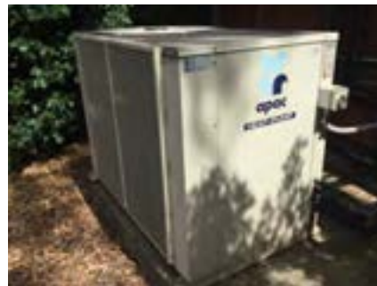
PHOTO NO.: J154351-001-PHOTO128 RESULT: ODS - POSITIVE BUILDING/LEVEL: B00B - GROUND LEVEL ROOM/LOCATION: EXTERIOR - VARIOUS THROUGHOUT FEATURE/MATERIAL: A/C UNIT - R22 - CHLORODIFLUOROMETHANE SAMPLE NO.: -
