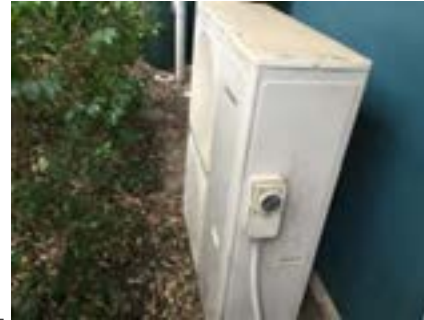
PHOTO NO.: J154351-001-PHOTO191 RESULT: ODS - POSITIVE BUILDING/LEVEL: B00K - GROUND LEVEL ROOM/LOCATION: EXTERIOR - SOUTH FEATURE/MATERIAL: A/C UNIT - R22 - CHLORODIFLUOROMETHANE SAMPLE NO.: -
