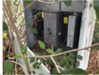
PHOTO NO.: J154351-001-PHOTO189 RESULT: ASBESTOS - PRESUMED POSITIVE BUILDING/LEVEL: B00B - GROUND LEVEL ROOM/LOCATION: EXTERIOR - WEST FEATURE/MATERIAL: ELECTRICAL - SWITCH BOARD - COMPRESSED BITUMINOUS ELECTRICAL PANEL SAMPLE NO.: NOT SAMPLED LIVE ELECTRICAL HAZARD
