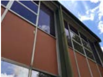
PHOTO NO.: J154351-001-PHOTO186 RESULT: ASBESTOS - POSITIVE BUILDING/LEVEL: B00D - ALL LEVELS ROOM/LOCATION: ALL AREAS - VARIOUS THROUGHOUT FEATURE/MATERIAL: INFILL PANELS - COMPRESSED CEMENT SHEETING SAMPLE NO.: PREVIOUSLY SAMPLED GREENCAP J146932-02-002-024
