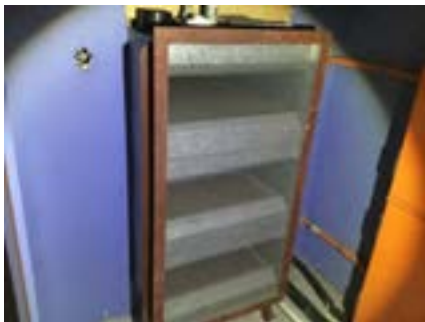
PHOTO NO.: J154351-001-PHOTO177 RESULT: SMF - POSITIVE BUILDING/LEVEL: B00D - GROUND LEVEL ROOM/LOCATION: DR0022 - PLANT ROOM - SOUTH FEATURE/MATERIAL: DUCTWORK INSULATION - INSULATION MATERIAL SAMPLE NO.: -
