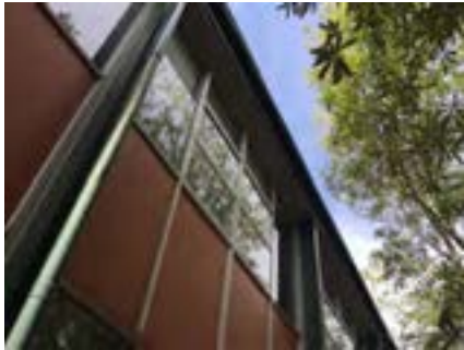
PHOTO NO.: J154351-001-PHOTO132 RESULT: ASBESTOS - PRESUMED POSITIVE BUILDING/LEVEL: B00B - LEVEL ONE ROOM/LOCATION: EXTERIOR - VARIOUS THROUGHOUT FEATURE/MATERIAL: EAVES - FIBRE CEMENT SHEETING SAMPLE NO.: NOT SAMPLED HEIGHT RESTRICTED
