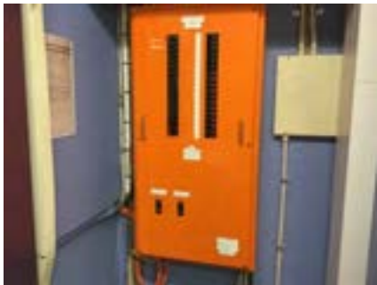
PHOTO NO.: J154351-001-PHOTO171 RESULT: ASBESTOS - PRESUMED POSITIVE BUILDING/LEVEL: B00D - GROUND LEVEL ROOM/LOCATION: DR0014 - ELECTRICAL CUPBOARD - WEST FEATURE/MATERIAL: ELECTRICAL - SWITCH BOARD - COMPRESSED BITUMINOUS ELECTRICAL PANEL SAMPLE NO.: NOT SAMPLED LIVE ELECTRICAL HAZARD
