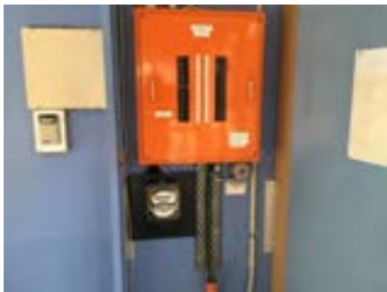
PHOTO NO.: J154351-001-PHOTO001 RESULT: ASBESTOS - PRESUMED POSITIVE BUILDING/LEVEL: B00K - GROUND LEVEL ROOM/LOCATION: KR0009 - ELECTRICAL CUPBOARD - EAST FEATURE/MATERIAL: ELECTRICAL - SWITCH BOARD - COMPRESSED BITUMINOUS ELECTRICAL PANEL SAMPLE NO.: NOT SAMPLED LIVE ELECTRICAL HAZARD
