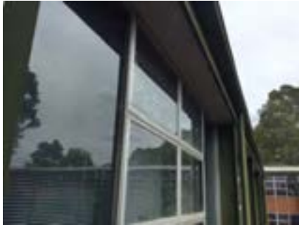
PHOTO NO.: J154351-001-PHOTO116 RESULT: ASBESTOS - PRESUMED POSITIVE BUILDING/LEVEL: B00E - LEVEL ONE ROOM/LOCATION: ALL AREAS - VARIOUS THROUGHOUT FEATURE/MATERIAL: EAVES - FIBRE CEMENT SHEETING SAMPLE NO.: NOT SAMPLED HEIGHT RESTRICTED
