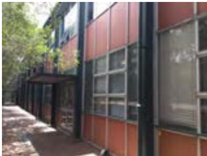
PHOTO NO.: J154351-001-PHOTO131 RESULT: ASBESTOS - POSITIVE BUILDING/LEVEL: B00B - ALL LEVELS ROOM/LOCATION: ALL AREAS - VARIOUS THROUGHOUT FEATURE/MATERIAL: INFILL PANELS - COMPRESSED CEMENT SHEETING SAMPLE NO.: PREVIOUSLY SAMPLED GREENCAP J146932-02-002-024
