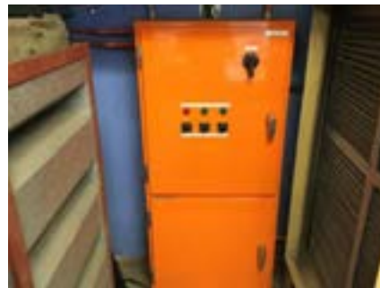
PHOTO NO.: J154351-001-PHOTO168 RESULT: ASBESTOS - PRESUMED POSITIVE BUILDING/LEVEL: B00D - GROUND LEVEL ROOM/LOCATION: DR0017 - PLANT ROOM - EAST FEATURE/MATERIAL: ELECTRICAL - SWITCH BOARD - COMPRESSED BITUMINOUS ELECTRICAL PANEL SAMPLE NO.: NOT SAMPLED LIVE ELECTRICAL HAZARD
