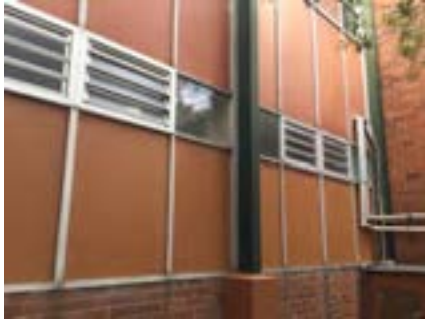
PHOTO NO.: J154351-001-PHOTO185 RESULT: ASBESTOS - POSITIVE BUILDING/LEVEL: B00D - ALL LEVELS ROOM/LOCATION: ALL AREAS - VARIOUS THROUGHOUT FEATURE/MATERIAL: INFILL PANELS - COMPRESSED CEMENT SHEETING SAMPLE NO.: PREVIOUSLY SAMPLED GREENCAP J146932-02-002-024
