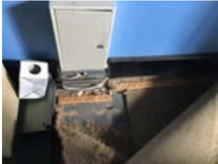
PHOTO NO.: J154351-001-PHOTO157 RESULT: ASBESTOS - POSITIVE BUILDING/LEVEL: B00D - GROUND LEVEL ROOM/LOCATION: DR0007 - SCANN/RECORDS STORAGE - THROUGHOUT FEATURE/MATERIAL: FLOOR COVERING - VINYL TILES & ADHESIVE SAMPLE NO.: J154351-001-049
