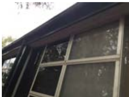
PHOTO NO.: J154351-001-PHOTO037 RESULT: ASBESTOS - POSITIVE BUILDING/LEVEL: B00A - GROUND LEVEL ROOM/LOCATION: EXTERIOR - VARIOUS THROUGHOUT FEATURE/MATERIAL: EAVES - FIBRE CEMENT SHEETING SAMPLE NO.: J154351-001-010
