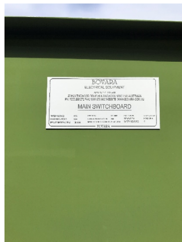
Figure 2 New Main Switchboard
