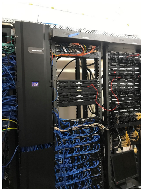
Figure 3 – Existing Communications Rack with Spare Capacity
