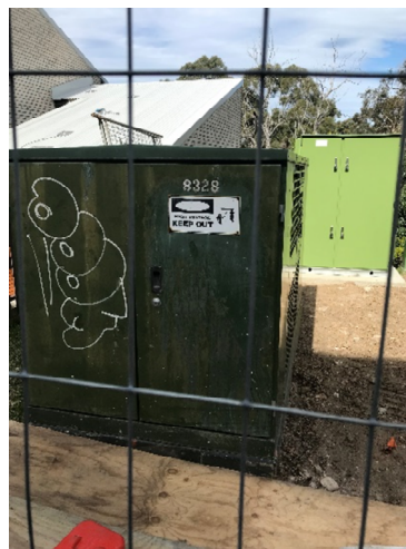
Figure 1 Existing Substation with New Main Switchboard
