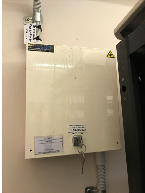
Figure 3 – Existing Street Fibre Incomer
