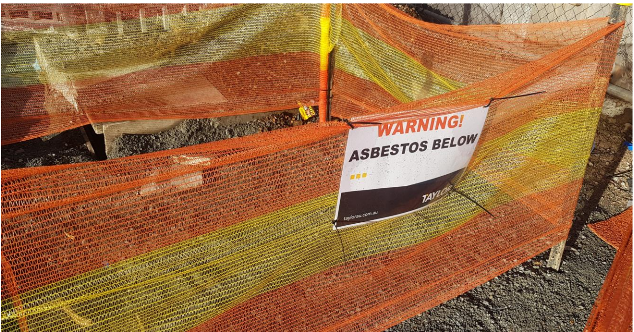
Photo 4: Identification of asbestos conduit.
