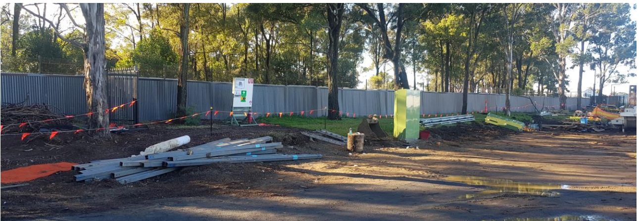
Photo 7: Tree protection not in place.
