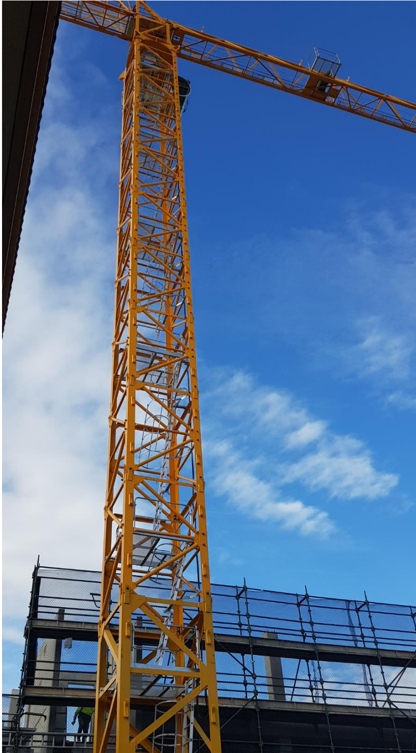
Photo 3: Tower crane. Note several complaints were received in relation to its erection
