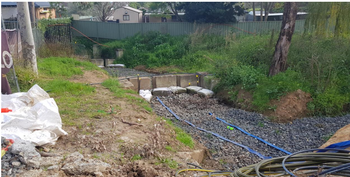
Photo 2: Rock filter dam
