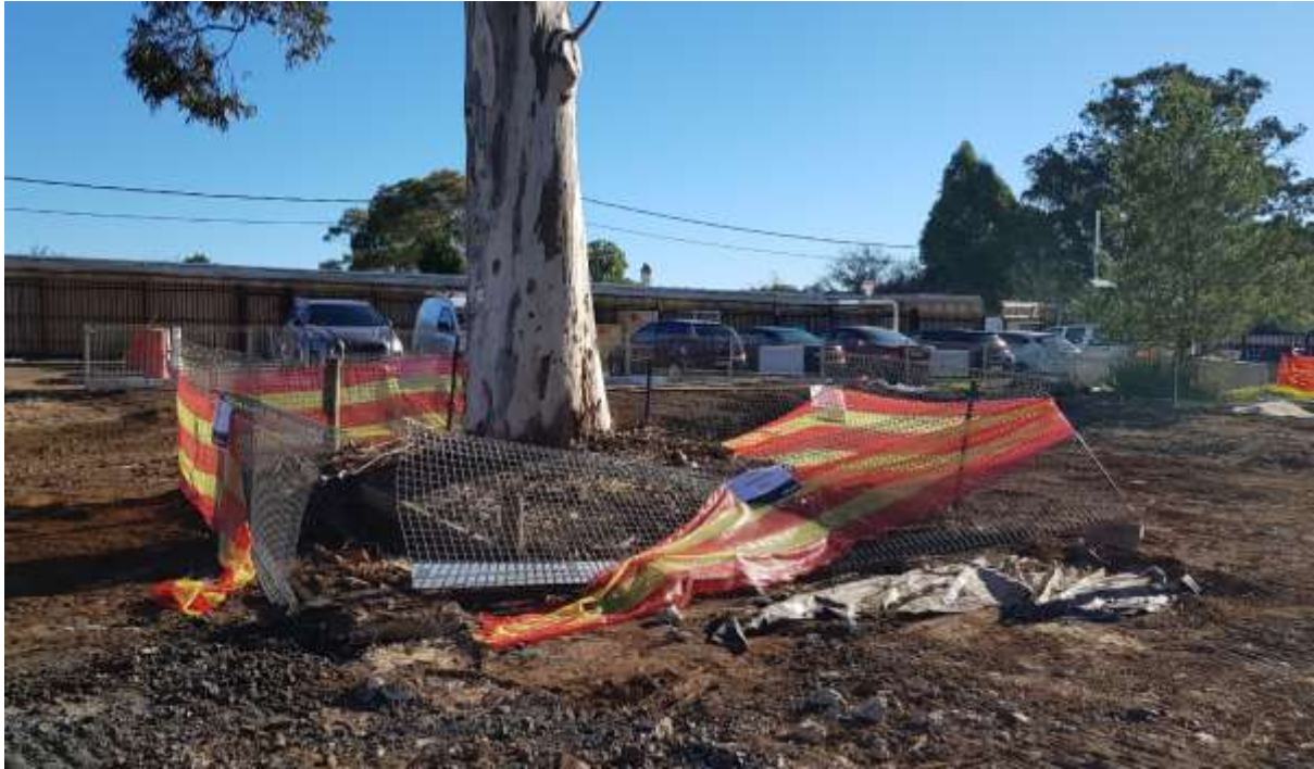
Photo 1: Tree Protection Zone not set at required diameter and damaged.
