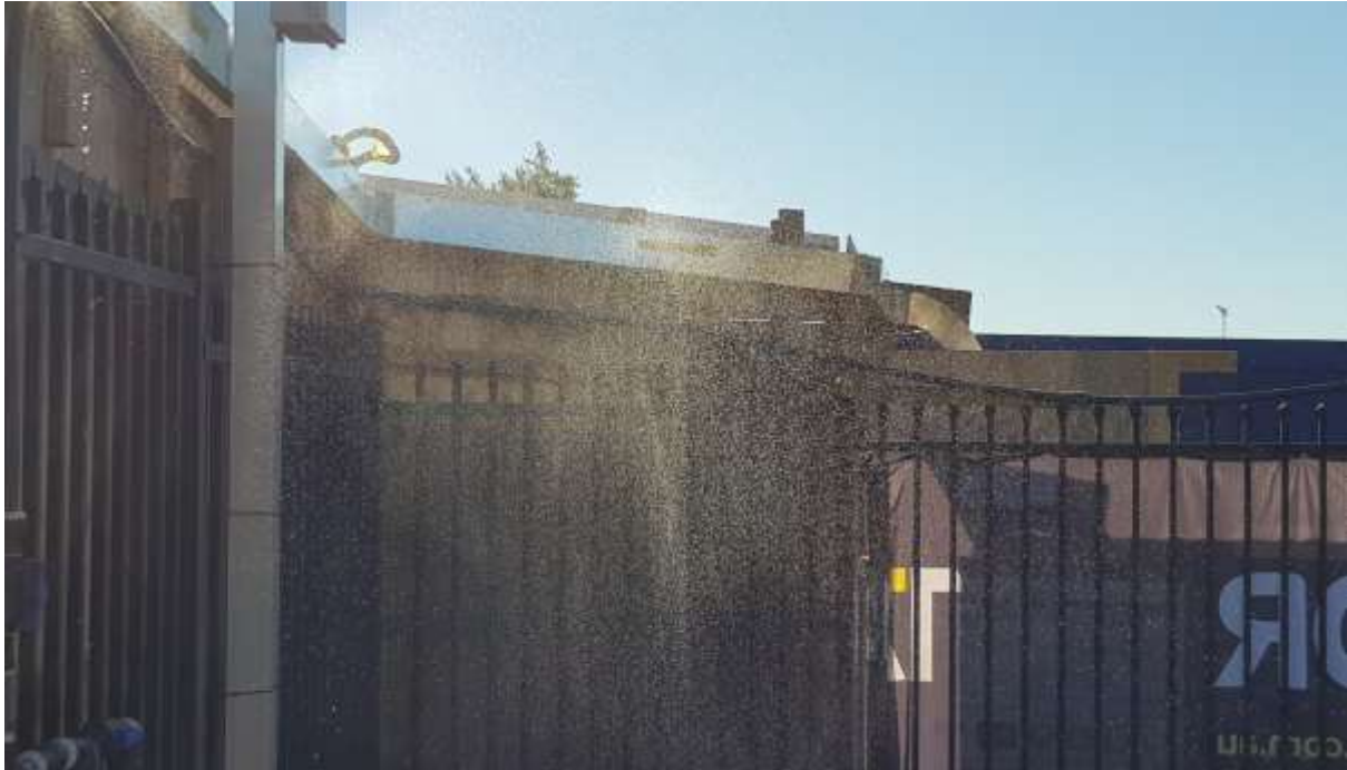
Photo 3: Boundary misting system
