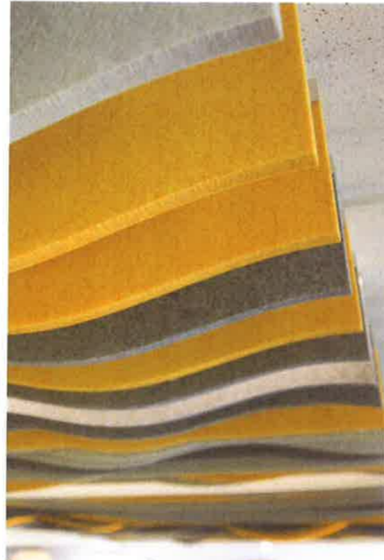
Acoustic baffle ceiling to maker spaces
