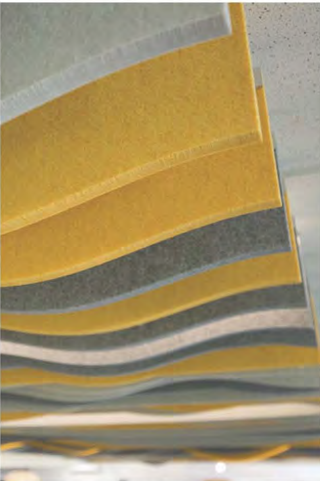
Aoustic baffle ceiling to maker spaces
