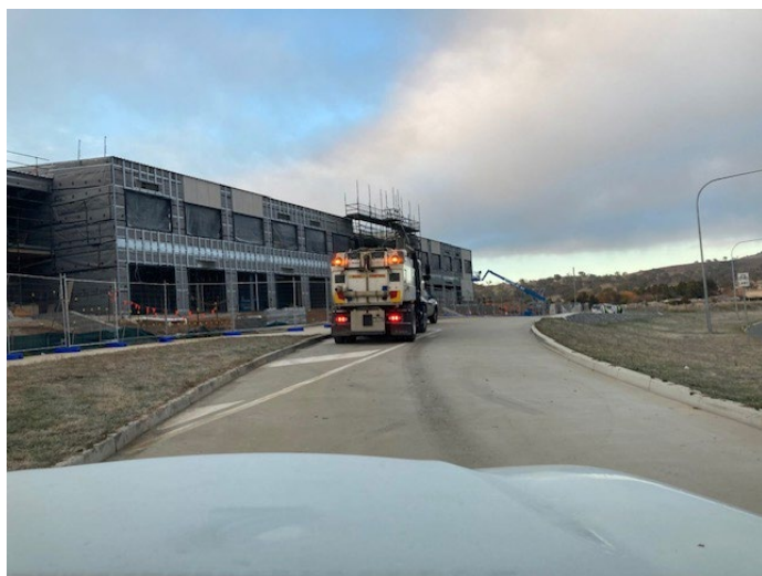
Evidence of Street Sweeper on site
