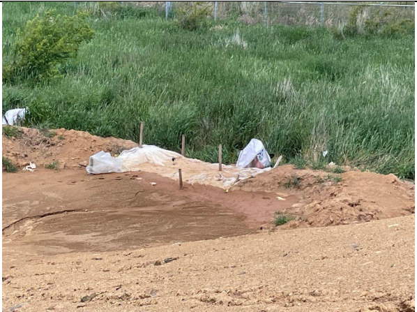
End of line sediment controls
