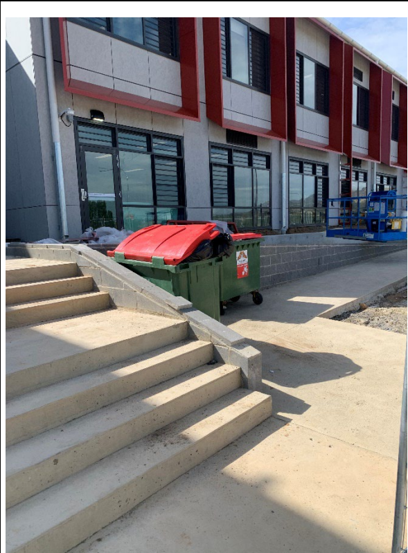
General waste bins (ready for service - lids closed)
