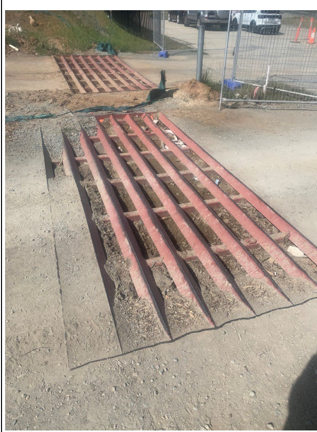
Rumble grid at vehicle access point
