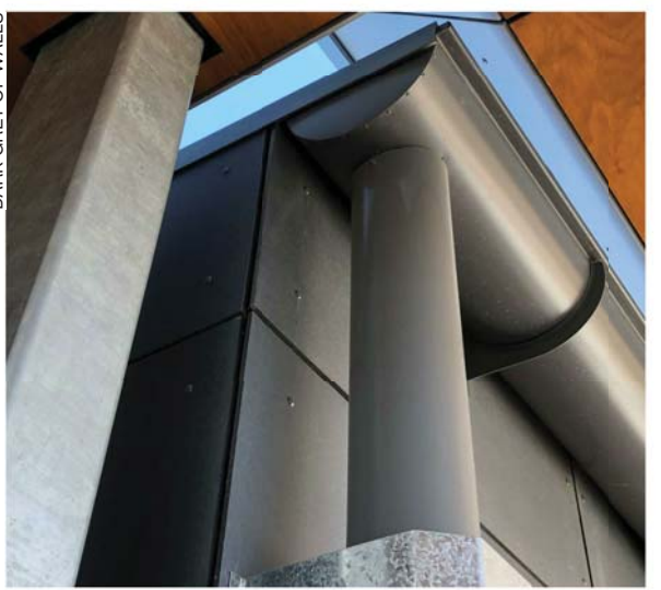
PREFINISHED METAL GUTTER AND FLASHING COLOUR TO MATCH DARK GREY OF WALLS
