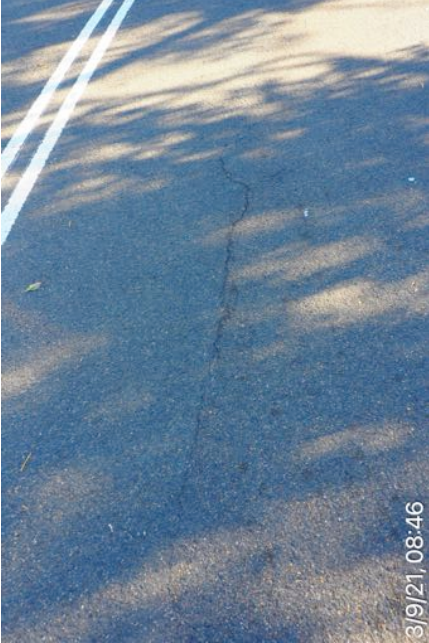
Gladstone Avenue Mosman Road surface from Keston to Avenue Road 3 September 2021 at 08:46:59
