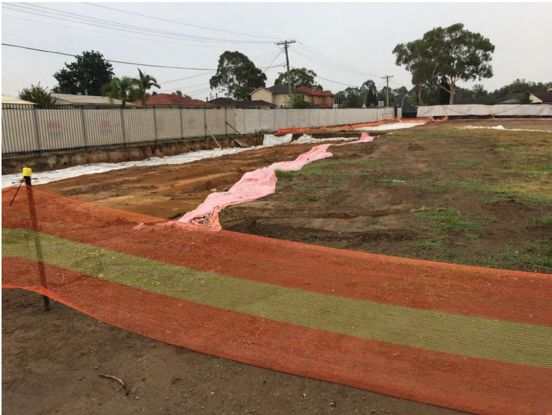
Photo 4: Part of Area 4 and Area 1 in the west of the site where excavation of contaminated soils has been completed
