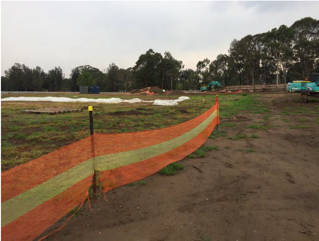
Photo 5: View from near the site compound looking towards the northeast corner of the site. Note the clean soil stockpiles and the two excavators (unused at the time of the inspection) in the background
