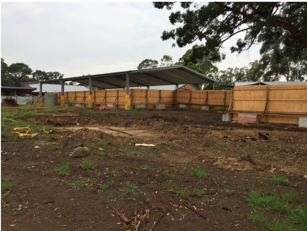
Photo 6: View looking southeast towards the Warwick Farm Public school, noting the hoarding that has been established to separate the school from the site
