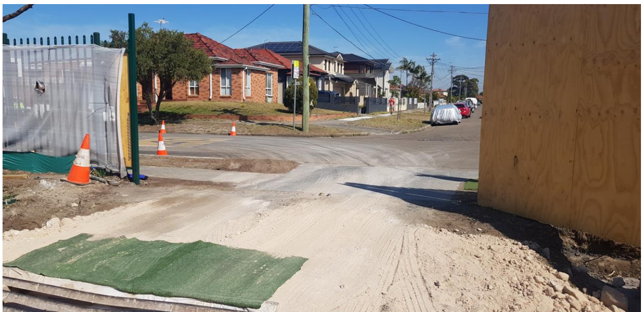
Photo 6: Tracking of dust on Beehag St and rumble grid in foreground during site inspection
