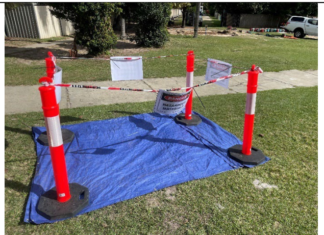
Photo 4: Covered trench with asbestos warning signage and tape
