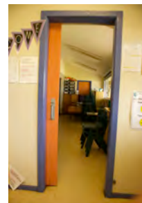
Photo #: IMG0021.jpg Caption: CR0008 - Looking into CR0005 doors open Camera Model: Canon EOS M50 Focal Length: 15.00mm Shutter Speed: 1/13
