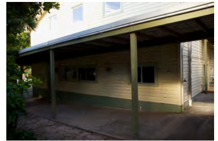
Photo #: IMG0150.jpg Caption: External - East towards CR9001 & CR9002 Camera Model: Canon EOS M50 Focal Length: 18.00mm Shutter Speed: 1/100
