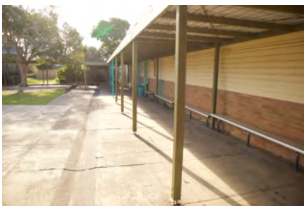
Photo #: IMG0106.jpg Caption: External - North west along southern side of western arm of building Camera Model: Canon EOS M50 Focal Length: 15.00mm Shutter Speed: 1/160
