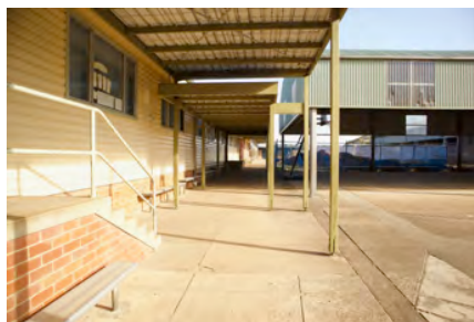
Photo #: IMG0107.jpg Caption: External - South along western side of southern arm of building Camera Model: Canon EOS M50 Focal Length: 15.00mm Shutter Speed: 1/200
