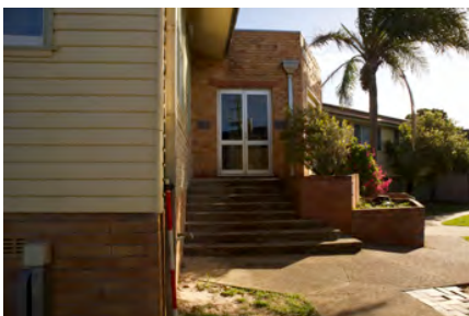
Photo #: IMG0130.jpg Caption: External - West towards CR0012 Camera Model: Canon EOS M50 Focal Length: 15.00mm Shutter Speed: 1/320
