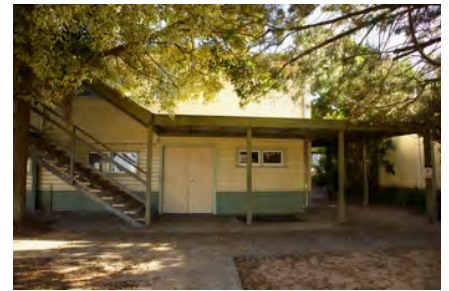
Photo #: IMG0162.jpg Caption: External - Southwest towards CR9003 Camera Model: Canon EOS M50 Focal Length: 15.00mm Shutter Speed: 1/125
