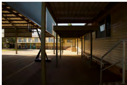
Photo #: IMG0116.jpg Caption: External - North along western side of southern arm of building Camera Model: Canon EOS M50 Focal Length: 15.00mm Shutter Speed: 1/250
