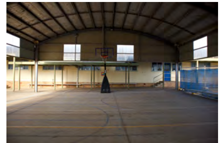
Photo #: IMG0114.jpg Caption: External - East towards CR0022 & CR0024 Camera Model: Canon EOS M50 Focal Length: 15.00mm Shutter Speed: 1/100
