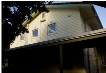
Photo #: IMG0149.jpg Caption: External - East towards CR0001 & CR0002 Camera Model: Canon EOS M50 Focal Length: 18.00mm Shutter Speed: 1/250
