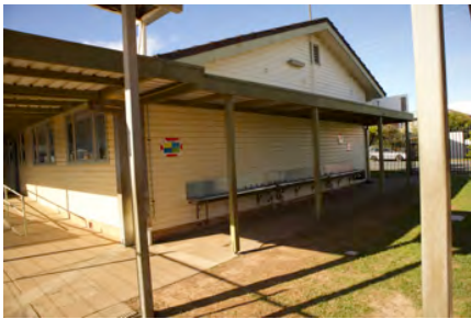
Photo #: IMG0148.jpg Caption: External - North east towards CR0030 Camera Model: Canon EOS M50 Focal Length: 15.00mm Shutter Speed: 1/320
