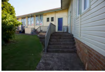
Photo #: IMG0134.jpg Caption: External - Southwest along southern side of CR0015 Camera Model: Canon EOS M50 Focal Length: 15.00mm Shutter Speed: 1/200
