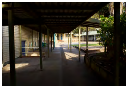
Photo #: IMG0119.jpg Caption: External - South east along southern side of western arm of building Camera Model: Canon EOS M50 Focal Length: 18.00mm Shutter Speed: 1/125
