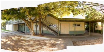
Photo #: IMG0160.jpg Caption: External - South towards CR9005 Camera Model: Canon EOS M50 Focal Length: 15.00mm Shutter Speed: 1/80
