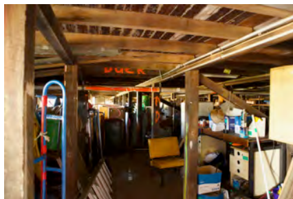
Photo #: IMG0164.jpg Caption: External - Southeast view of CR9005 Camera Model: Canon EOS M50 Focal Length: 15.00mm Shutter Speed: 1/0
