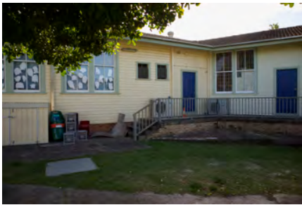
Photo #: IMG0136.jpg Caption: External - Northwest towards CR0018 Camera Model: Canon EOS M50 Focal Length: 15.00mm Shutter Speed: 1/250
