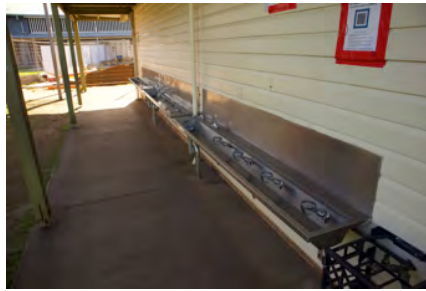
Photo #: IMG0146.jpg Caption: External - Detail of drinking trough along southern side of CR0030 Camera Model: Canon EOS M50 Focal Length: 15.00mm Shutter Speed: 1/200
