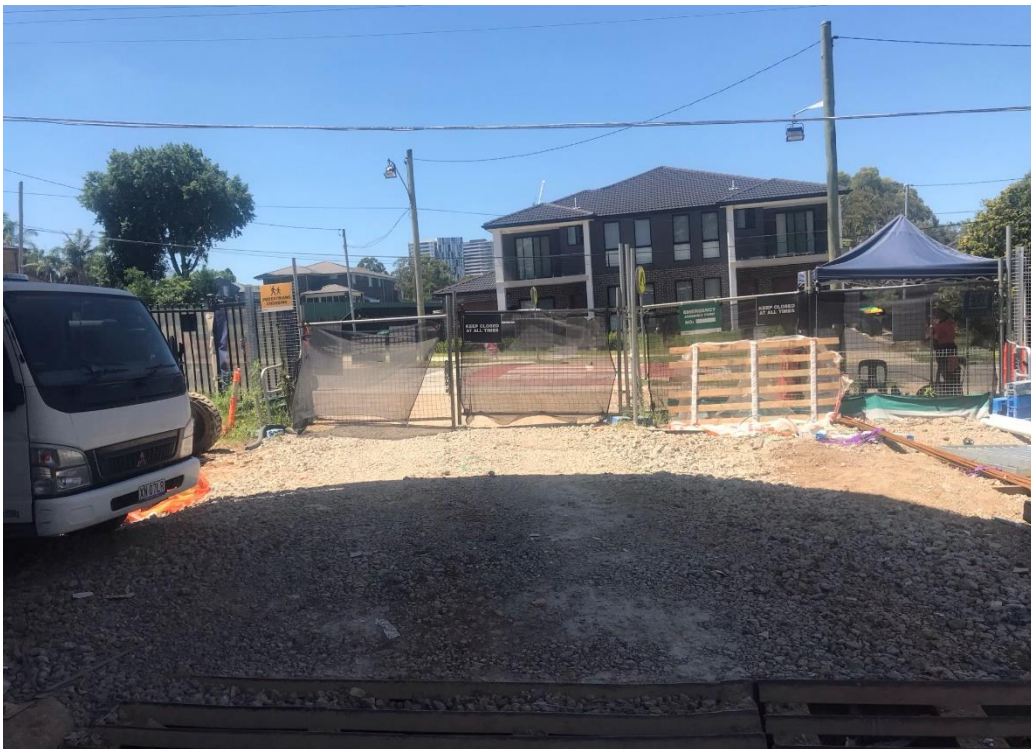
Figure 2: Gravel placed at entrance to prevent tracking of mud onto public roads
