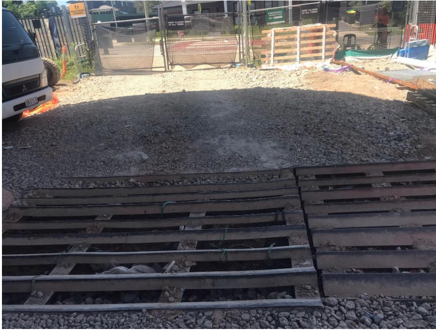
Figure 4: Gravel placed at site entrance to prevent tracking of mud onto public roads
