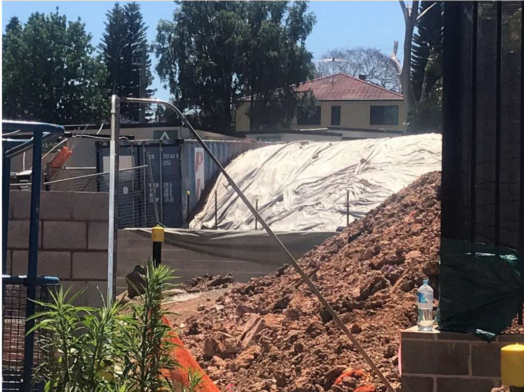
Figure 7: Stockpile at rear of site covered in geofabric and sediment fence in place around the perimeter of the site
