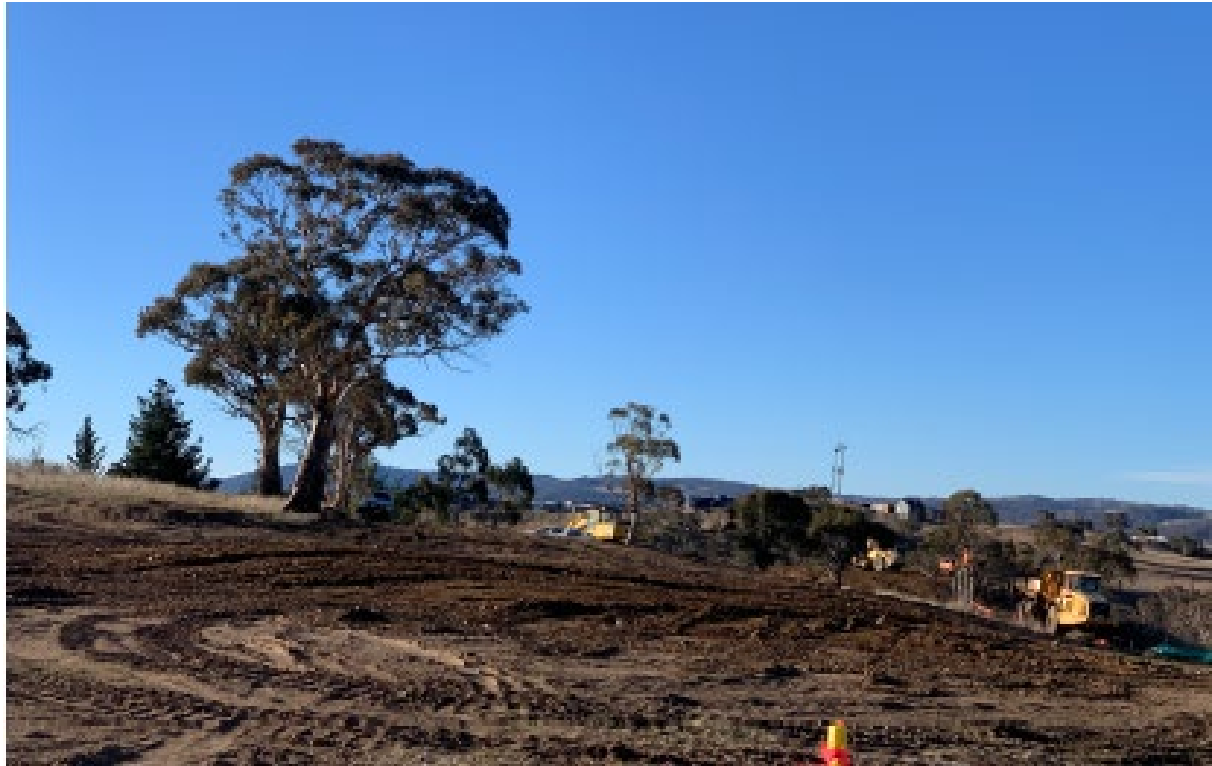
Figure 2-10 Construction of the Dry Jump and Ski Jump to north-east of site within JSRC Source: Blackash Bushfire Consulting
