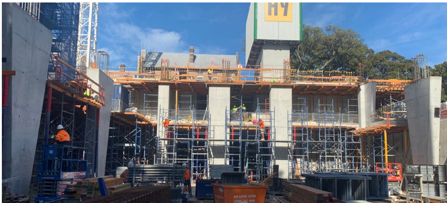
The triangular concrete pylons (right and left) that will support the floors above the indoor basketball court
