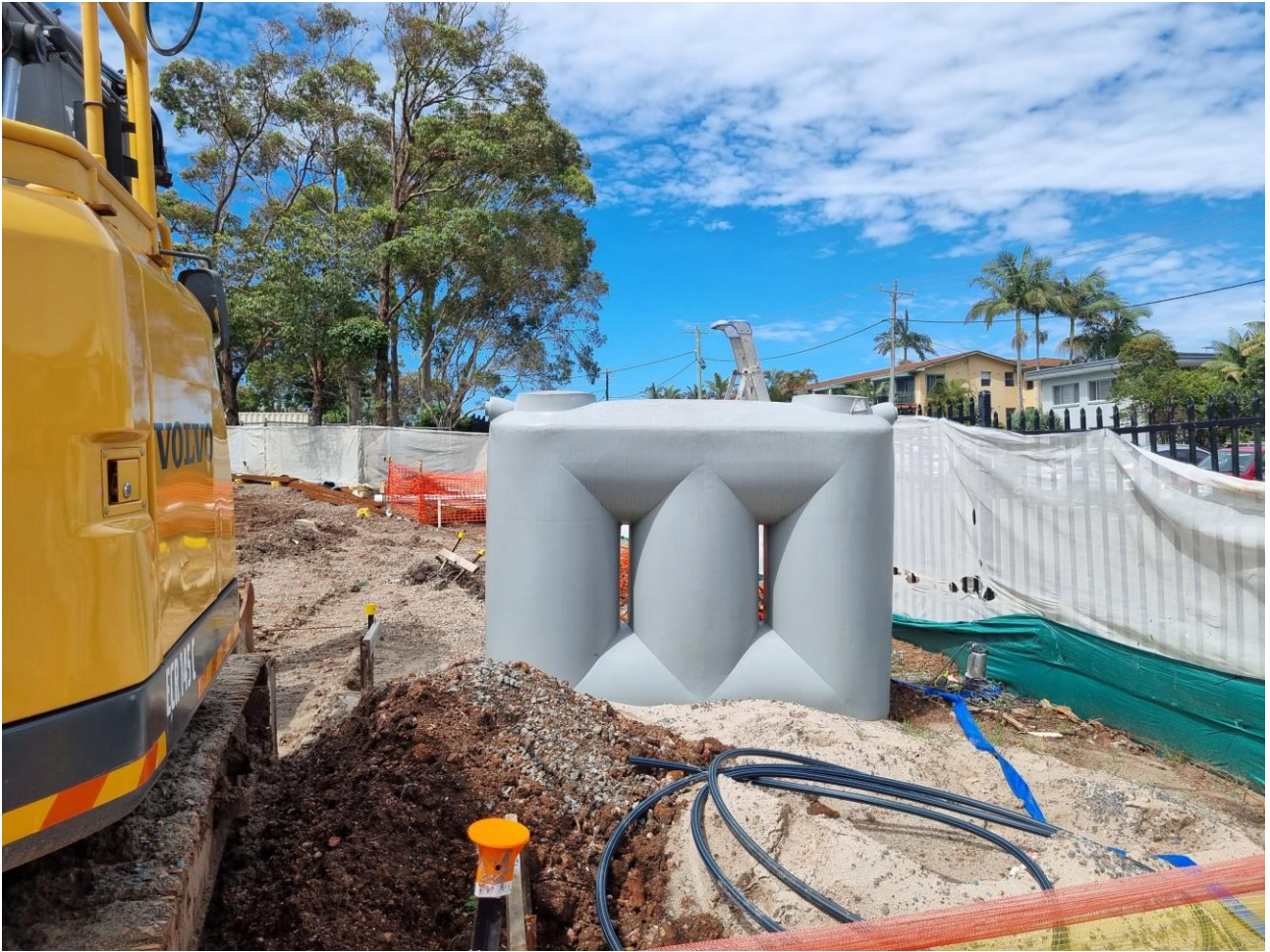
Plate 6 – PVC tank used for storage of site stormwater prior to tankering off site
