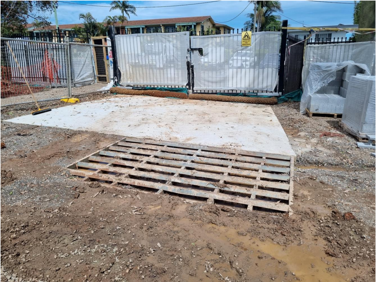
Plate 7 - Rumble grid and concrete pad used for cleaning wheels prior to exiting site
