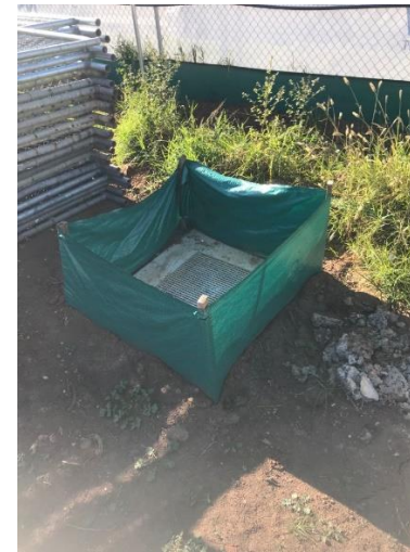
Photo 14 – Stormwater Pit Protection
