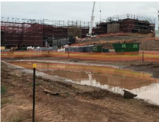
Photo 6 – Sedimentation Basin – needs to be maintained i.e. desilting
