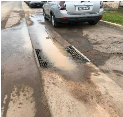
Photo 3a – Pit cover to be replaced and maintained.
