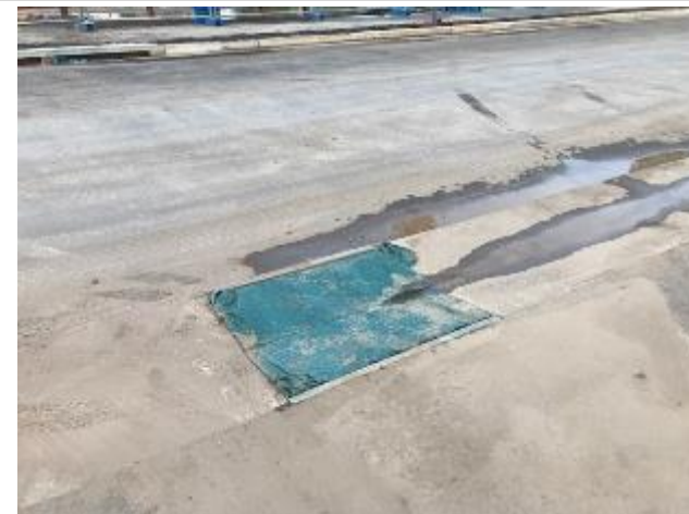
Photo 3b – Pit cover was rectified immediately upon issue noted by auditor.
