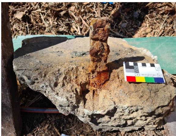
Figure 23. Concrete with iron pin removed from in between pans (provided by Curio Projects)
