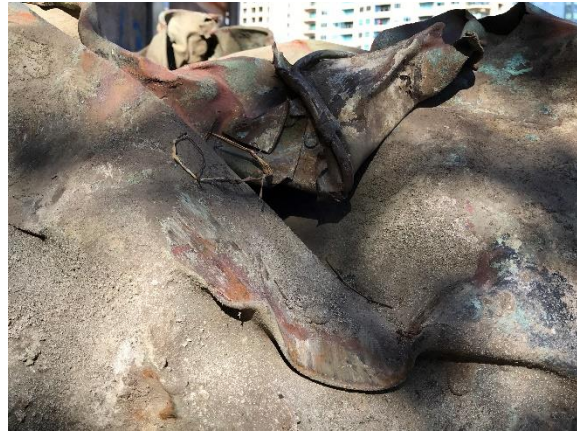
Figure 20. Detail of severe crumpling and folding of pan wall
