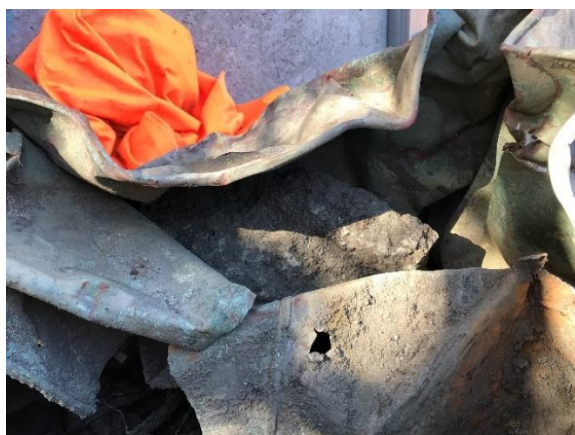
Figure 15. Concrete debris inserted between inner and outer pans. Hole punched through pan wall below
