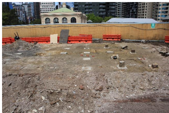
Figure 6-29. View south towards Surgeon’s Cottage showing exposed contexts (4.004), (5.002) and (6.001) following the removal of demolition contexts (1.001) and (4.001).
