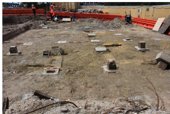
Figure 6-31. Overview of the Surgeon’s Cottage excavation area showing exposed concrete pads associated with Phase 6 school building and partially removed demolition fill (1-001). View east.
