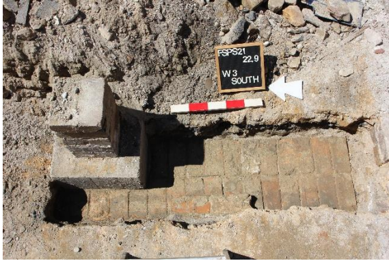
Figure 6-19. Detail of partially exposed Wall 3 footing (eastern elevation of the Cottage's verandah) sitting below an EEC Building concrete support pad and demolition fill (1.001).
