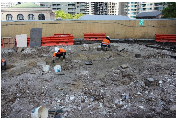
Figure 6-28. View south towards Surgeon’s Cottage excavation area. Unstratified fills and demolition contexts (1.001) and (4.001) visible across the site.
