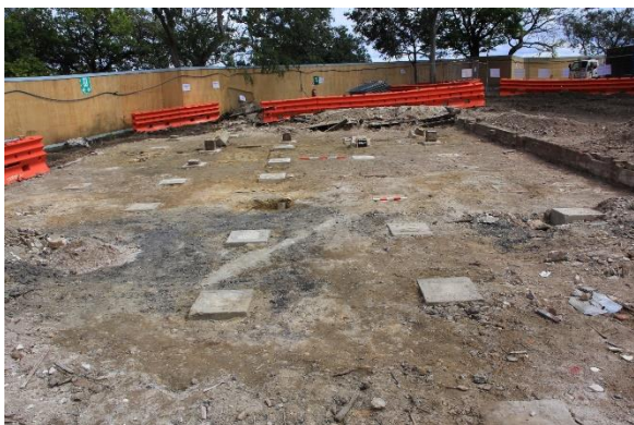
Figure 6-30. Overview of the Surgeon’s Cottage excavation area showing exposed concrete pads associated with the EEC Building (Phase 6) and partially removed demolition fill (1-001). View west.
