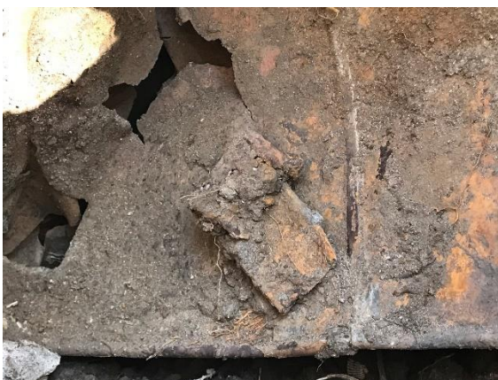
Figure 12. Detail of damaged strut, and tears in the metal
