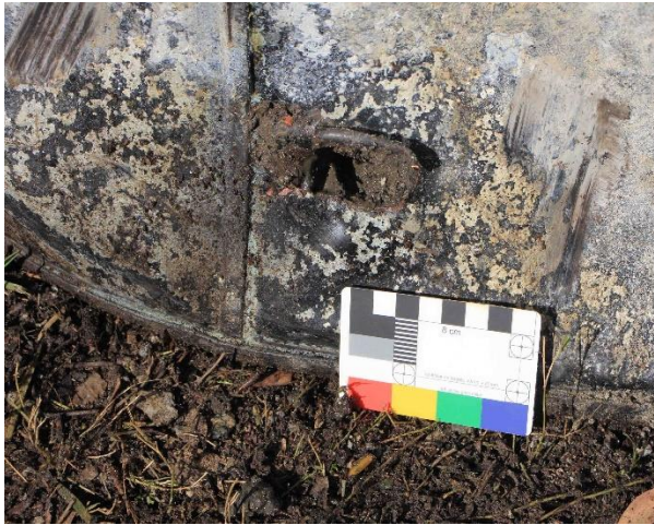
Figure 6-7 Detail of side seam and base seam. Note the puncture in the body.
