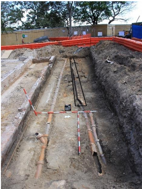
Figure 6-38. View west towards the northern elevations of the former EEC Building, the heavily truncated Surgeon Cottage's northern elevation (outlined in black) and a series of earthenware pipes (Phase 5 and/or 6) running north-south and east-west between footings for each former structure. View west.
