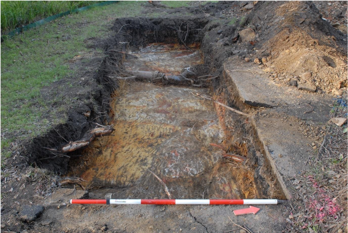
Figure 2-8. Test Trench 5 after excavation showing 5.005 (CEW pipe) and 5.008 (bedrock) exposed in trench. Source: Curio, 2019.
