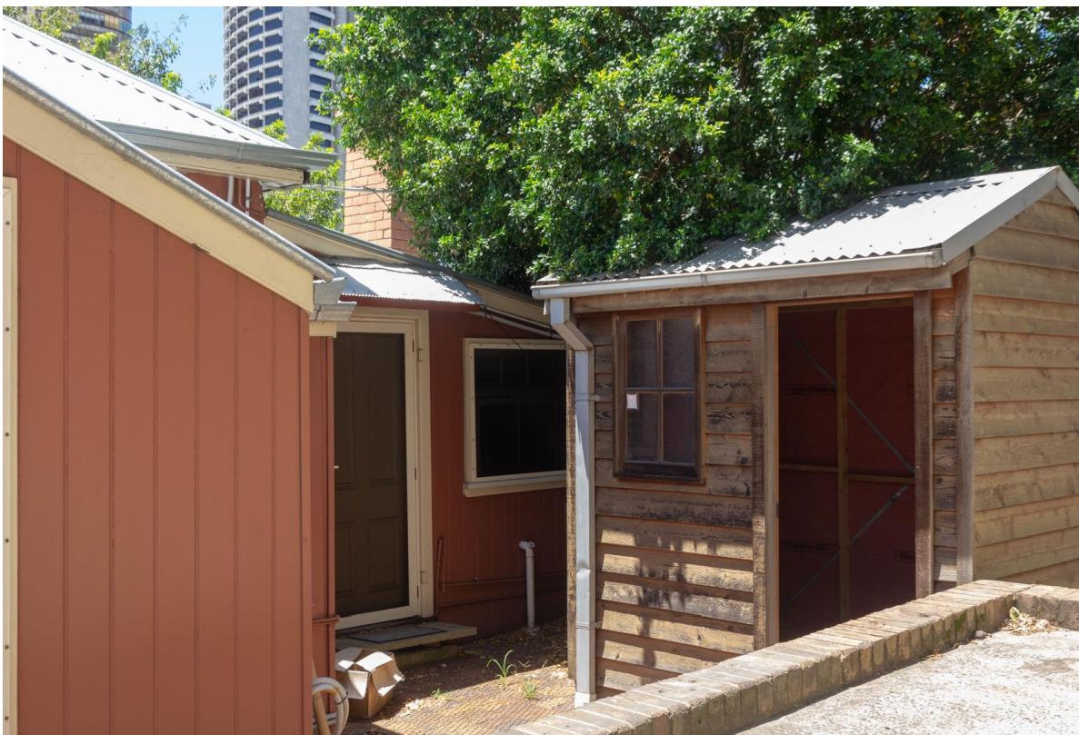
Figure 5-19: Former late addition non-significant weatherboard shed demolished as part of the 2023 works. (Source: Curio Projects)
