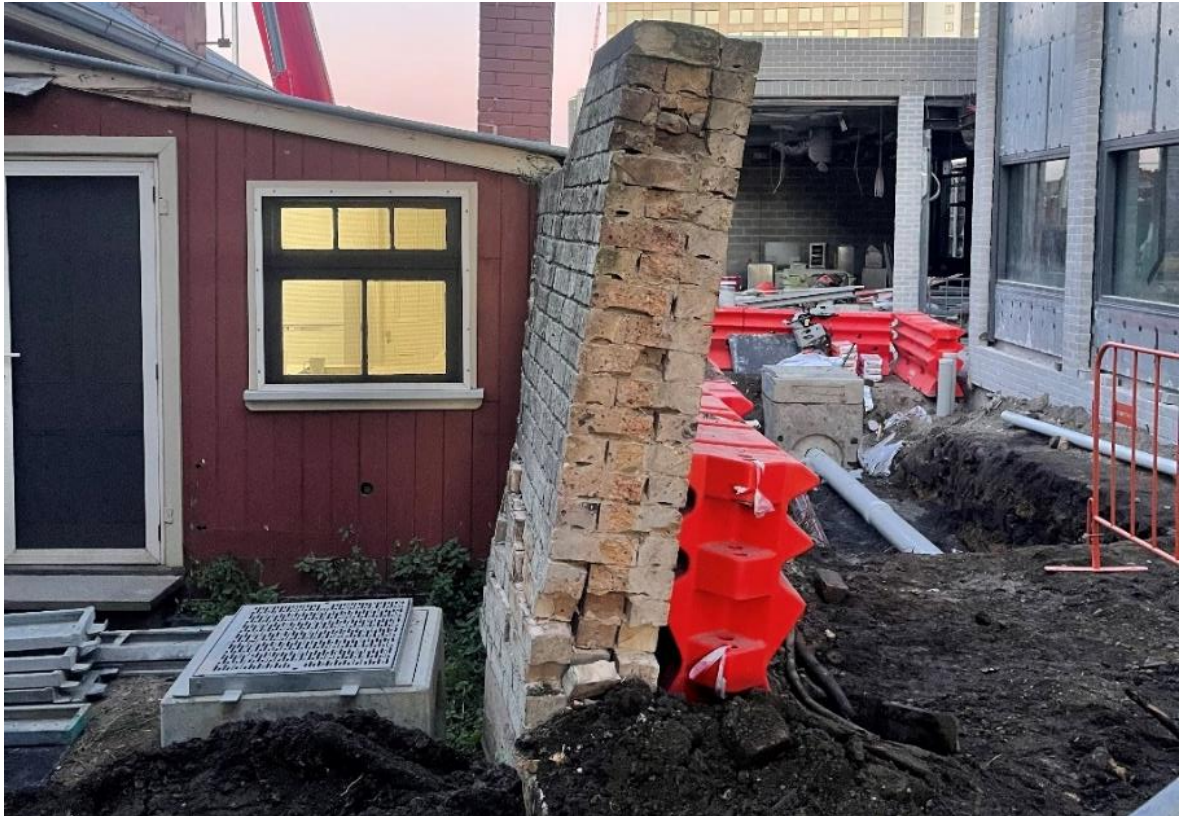
Figure 5.17: An example of a compromised section of the Wall -East Elevation pre-reconstruction (Curio Projects 2023)
