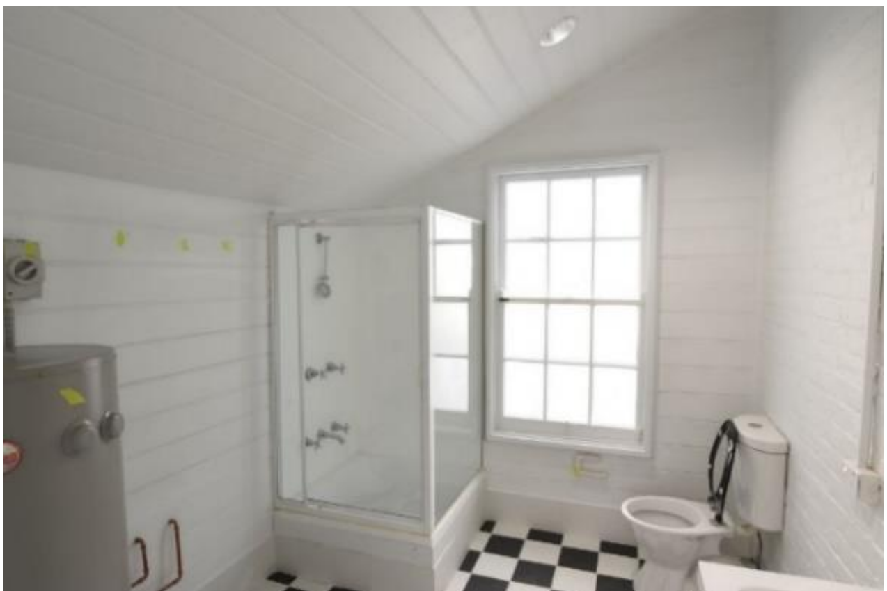
Figure 5-28: Image of bathroom (WC), with minor updates to paintwork, fixtures and fittings. Retains pre-2023 shower, flooring and sink.
