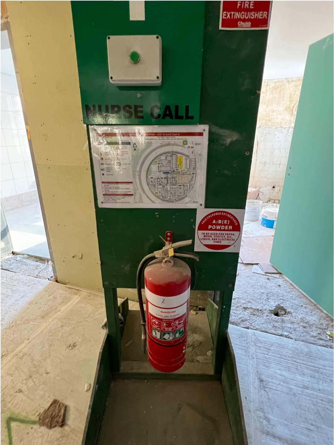
Figure 14 Fire extinguisher and associated safety signage at emergency station
