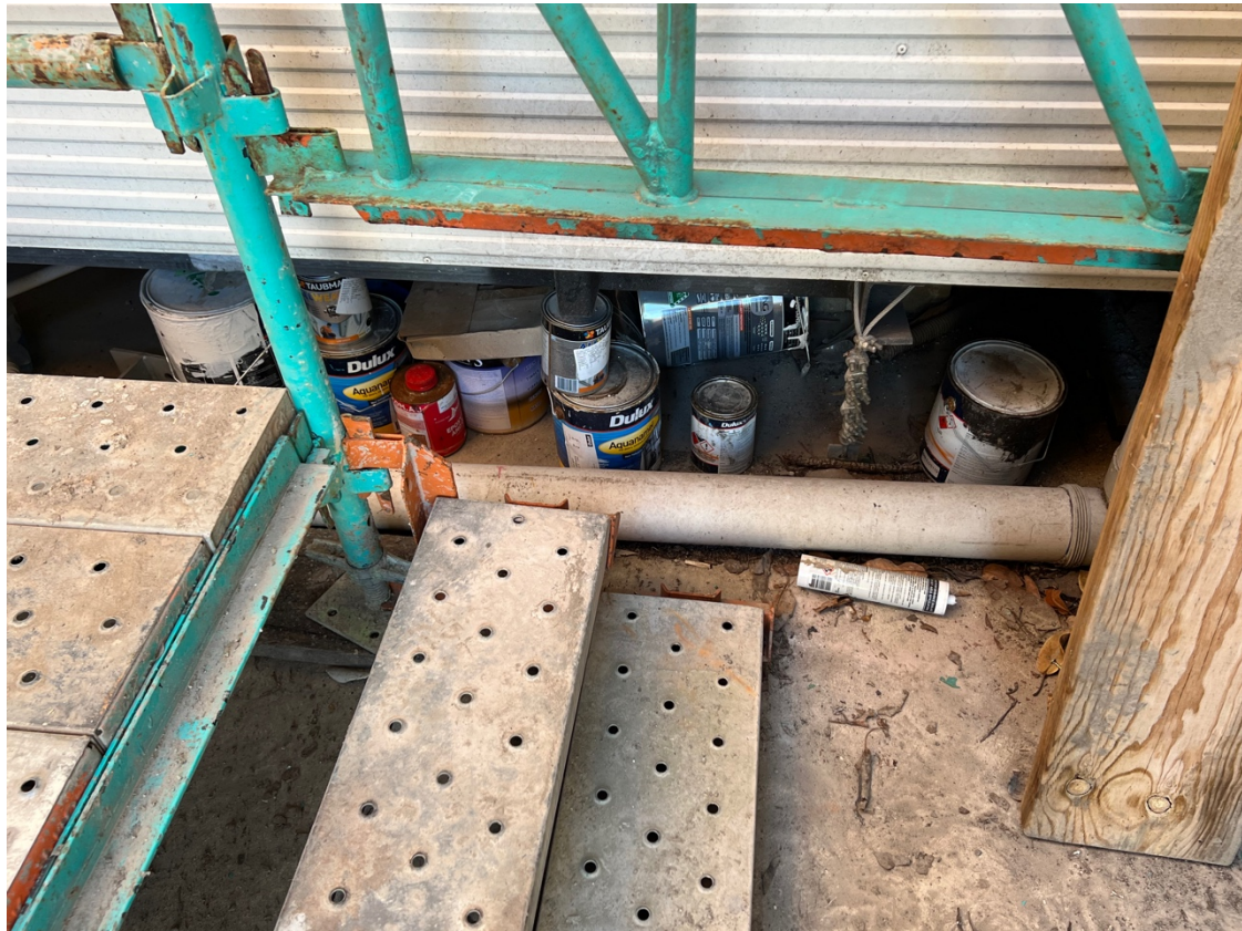
Figure 25 Stowage of flammable materials under site shed
