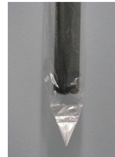
Figure 10 - positioning of pipe and foam plug at the bottom of plastic sleeve
