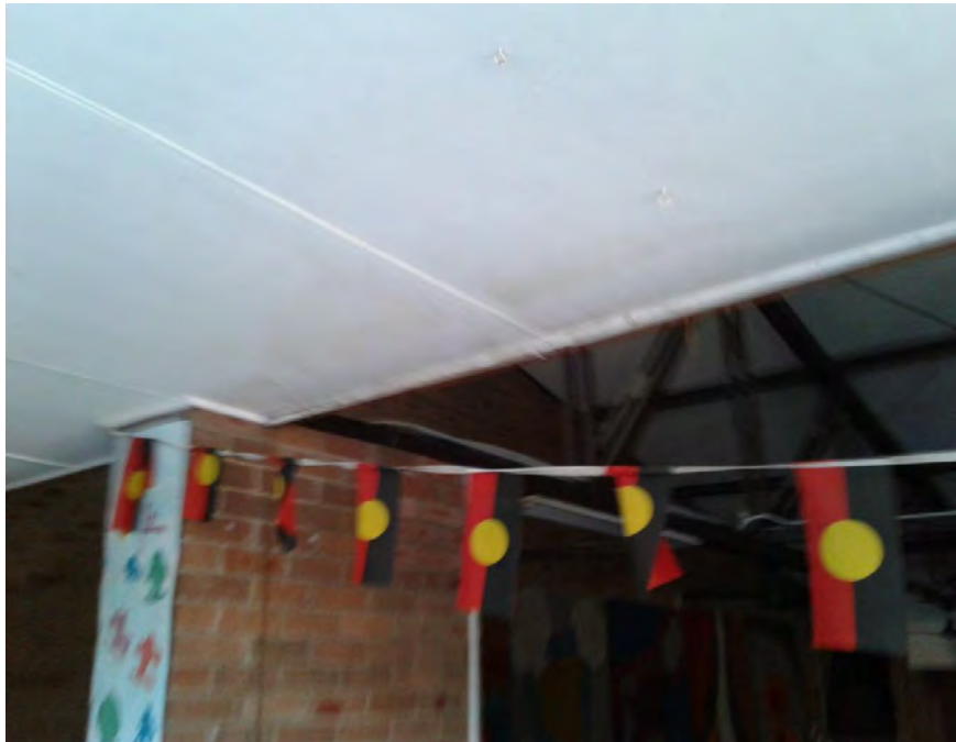
Photograph 37: B00C - R0025, Interior, Brick column, Dust above column, elevated lead (>0.5 mg/m2).
