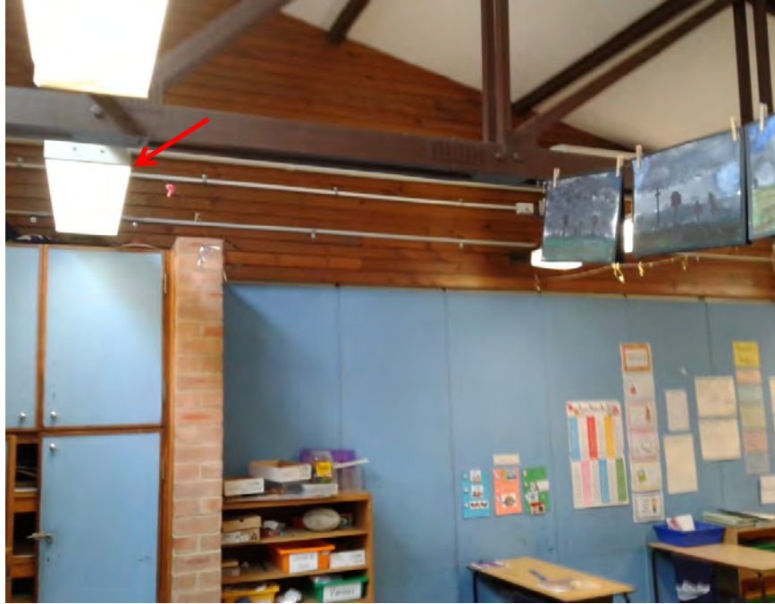
Photograph 26: B00B - R1003, Interior, Light fitting, Dust above light fitting, elevated lead (>0.5 mg/m2).
