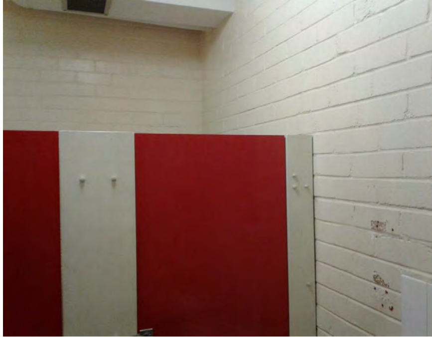
Photograph 9: B00A - R0021, Interior, Partitions in toilet, Compressed FCS sheeting, asbestos detected by analysis.
