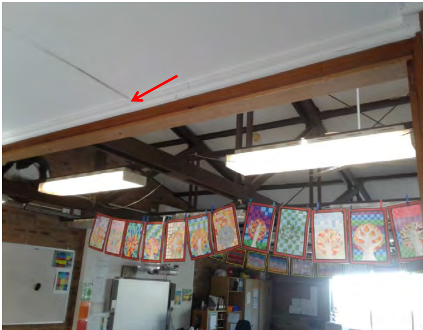
Photograph 29: B00B - R1014, Interior, Ceiling structure, White Flaking Paint, non-lead paint ( \leq 0.1\% lead w/w).
