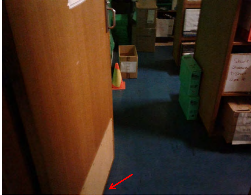
Photograph 13: B00A - R0032, Interior, Flooring material, Vinyl tiles under flooring, asbestos detected by analysis.
