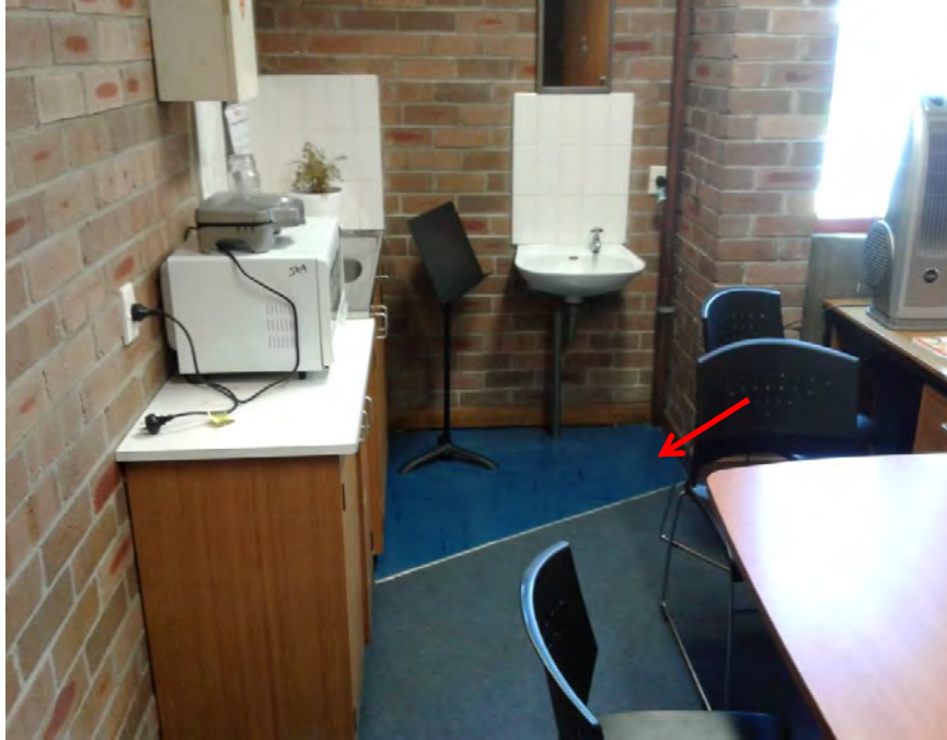
Photograph 3: B00A - R0006, Interior, Flooring material, Vinyl tiles, no asbestos detected by analysis.
