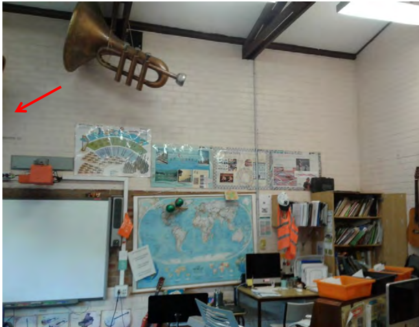
Photograph 14: B00A - R1001, Interior, Brick walls, Beige paint, non-lead paint ( \leq 0.1\% lead w/w).
