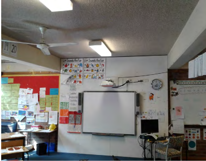
Photograph 24: B00B - R1002, Interior, Flooring material, Vinyl tiles under flooring, asbestos detected by analysis.
