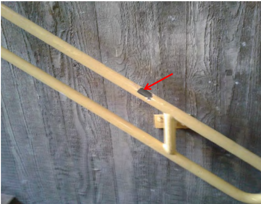
Photograph 8: B00A - R0019, Interior, Hand rails on stairs, Yellow paint, non-lead paint ( \leq 0.1\% lead w/w).
