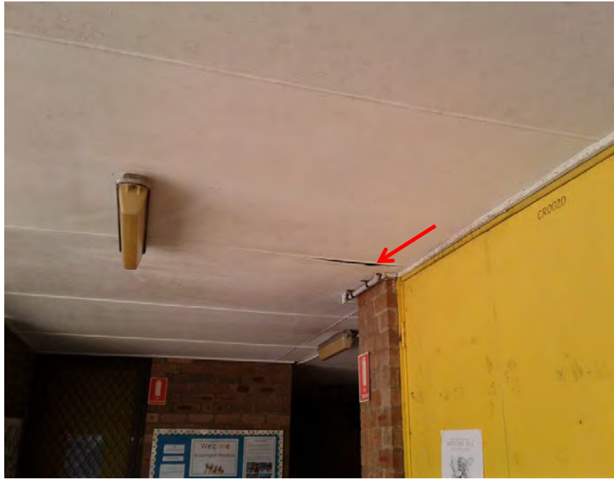
Photograph 32: B00C - R0005, Interior, Ceiling structure, FCS sheeting, no asbestos detected by analysis.
