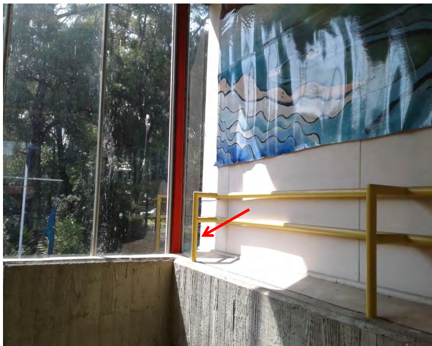
Photograph 21: B00B - R0025, Interior, FCS sheeting on wall, FCS sheeting, no asbestos detected by analysis.
