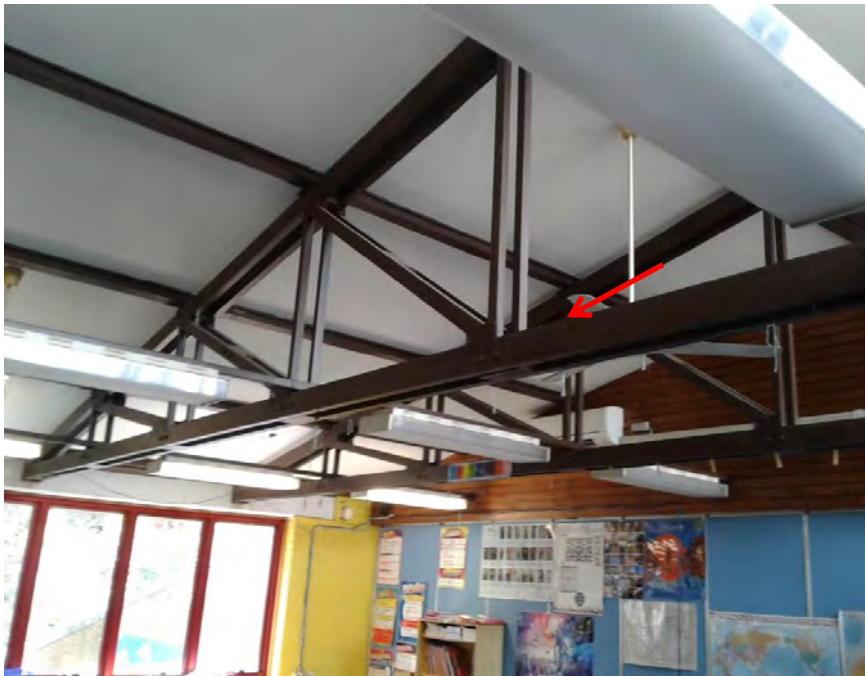
Photograph 27: B00B - R1008, Interior, Timber rafters, Brown paint, non-lead paint ( \leq 0.1\% lead w/w).
