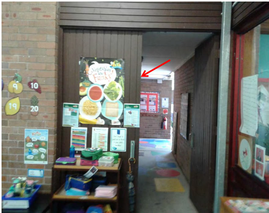
Photograph 31: B00C - R0002, Interior, Timber door frame, Brown Paint, non-lead paint ( \leq 0.1\% lead w/w).
