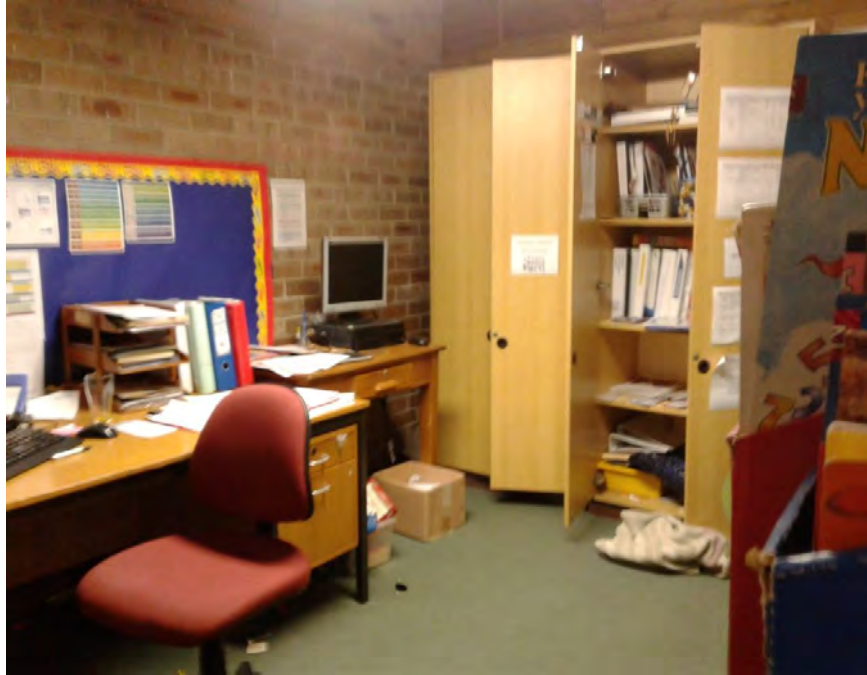
Photograph 38: B00C - R0029, Interior, Flooring material, Vinyl tiles under flooring, no asbestos identified visually.
