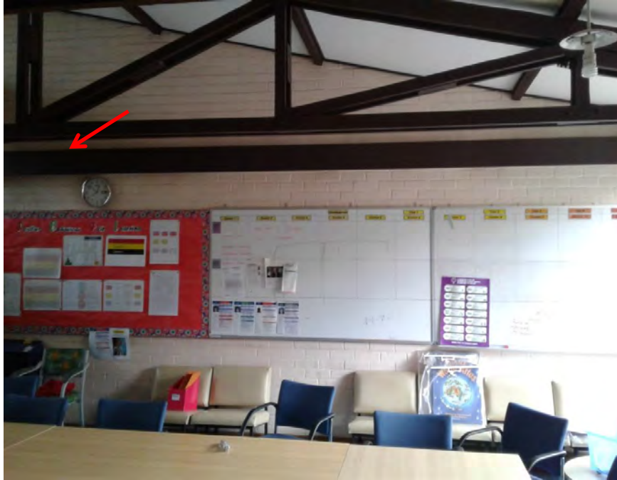
Photograph 15: B00A - R1002, Interior, Timber rafters, Dust above rafters, elevated lead (>0.5 mg/m 2 ).
