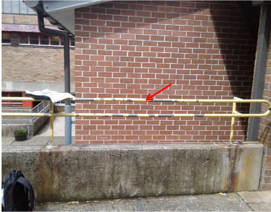
Photograph 36: B00C - R0024, Exterior, Hand rails, Yellow Paint, lead paint (>0.1% lead w/w).
