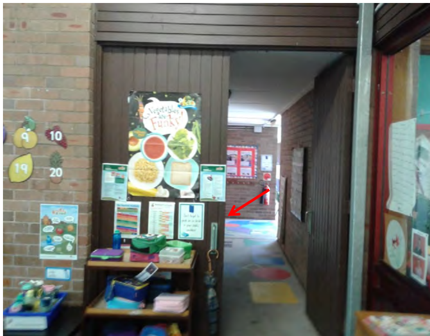
Photograph 39: B00C - R0034, Interior, Timber door, Brown Paint, non-lead paint ( \leq 0.1\% lead w/w).
