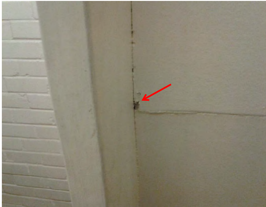
Photograph 10: B00A - R0022, Interior, Partitions in toilet, Compressed FCS sheeting, asbestos detected by analysis.
