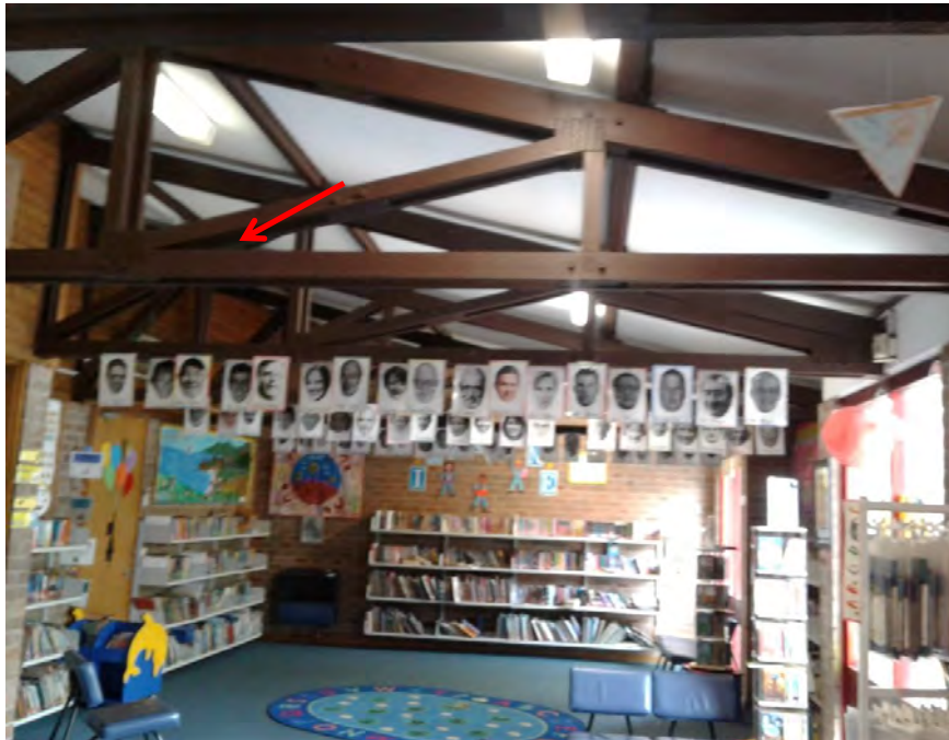
Photograph 16: B00A - R1003, Interior, Timber rafters, Brown paint, non-lead paint ( \leq 0.1\% lead w/w).
