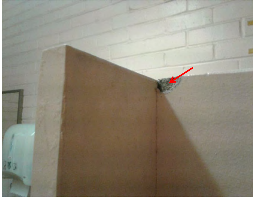
Photograph 19: B00A - R1019, Interior, Partitions in toilet, Compressed FCS sheeting, asbestos detected by analysis.
