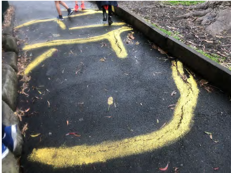
Plate 5: Image showing surface roots from Tree 20. P. Vezgoff
