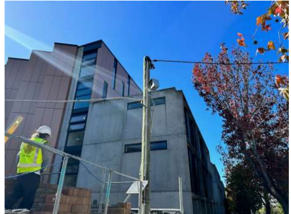
Photo 6: On site security camera
