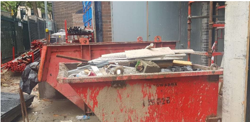
Photo 18: Bins in place near front boundary, some slurry observed
