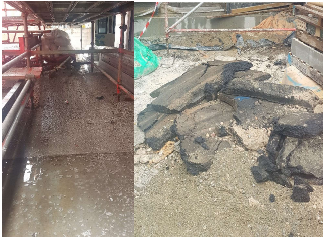
Photo 20: Some runoff/ concrete slurry under scaffold; small stockpile
