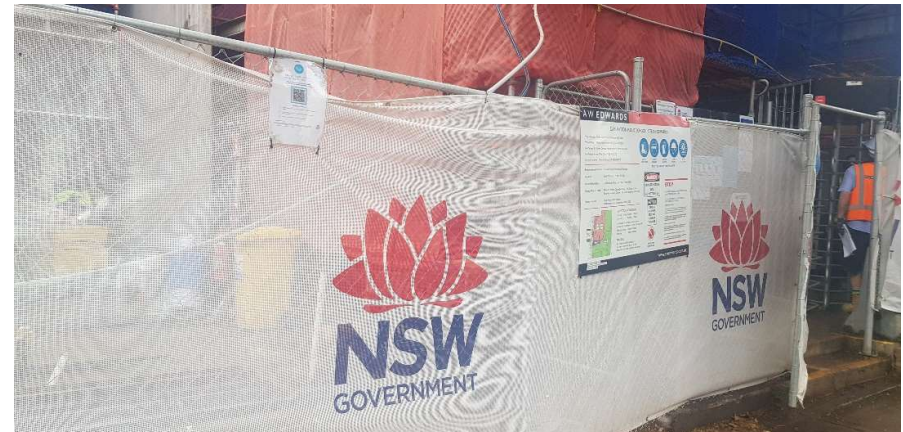
Photo 23: Government branded shade cloth, site notice observed.
