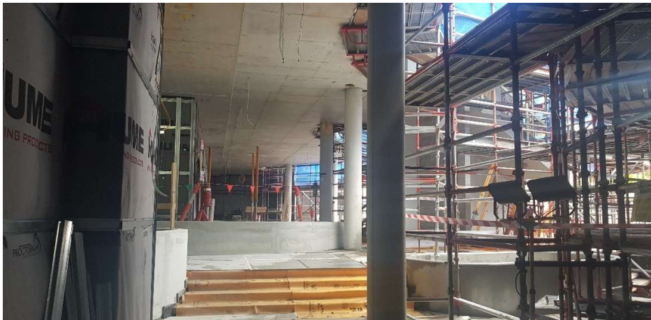
Photo 11: Ground floor, beside proposed library. Various levels observed
